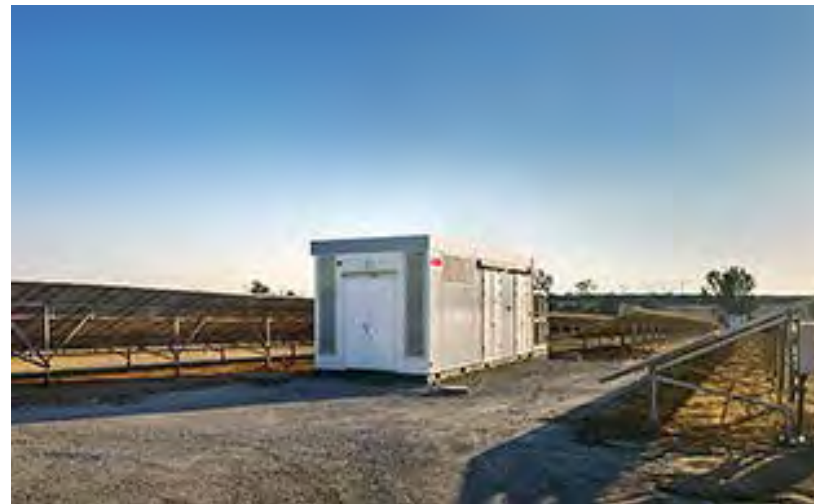
Figure 3.3 Inverter building (top) and typical Battery Storage (bottom)
