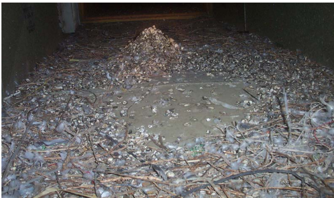
Figure 13. Droppings and feathers found in an air duct of a public school. Buildup can be a severe problem for building owners as droppings and feathers can contaminate vents of buildings, as well as food destined for human consumption. Droppings can also lead to structural damage from the high uric acid content; bacteria, fungal agents and parasites in the droppings also pose a health risk. Photo by Greg Ballard.
