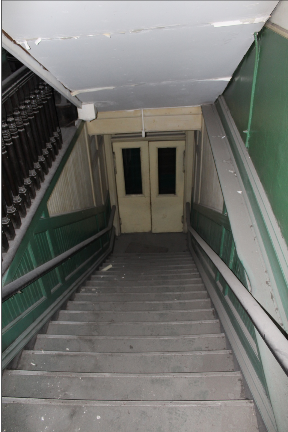
Plate 18 – Fortune Block, 232 Main Street, south end staircase giving access from Main Street to second and third floors, 2015. (M. Peterson, 2015.)
