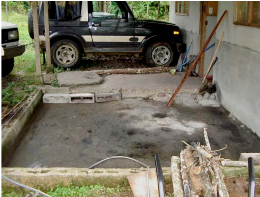
The front porch after some cleaning and just prior to beginning the process of pouring cement.
