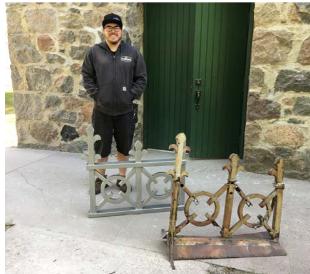
Top Right: Worker repairing the masonry exterior of the Old Stone Church. Center: Detail of damage to the stone pinnacle. Bottom Right: P2 Industries replica next to original roof ornament.
