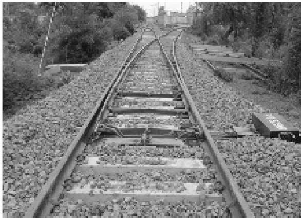
JHP: Old Point No. 106 on wooden sleepers converted to Point No. 338 on PSC sleepers
