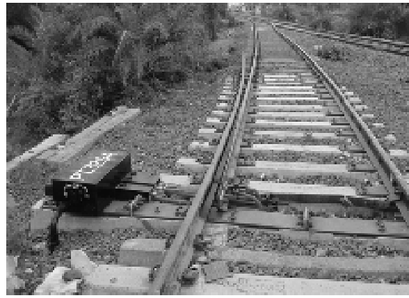
JHP: Old Point No. HP-1 on wooden sleepers converted to Point No. 330 on PSC sleepers
