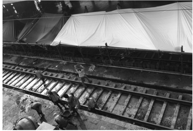
PF-5: Tarpaulins used to protect and preserve the quality of the green concrete during monsoon
