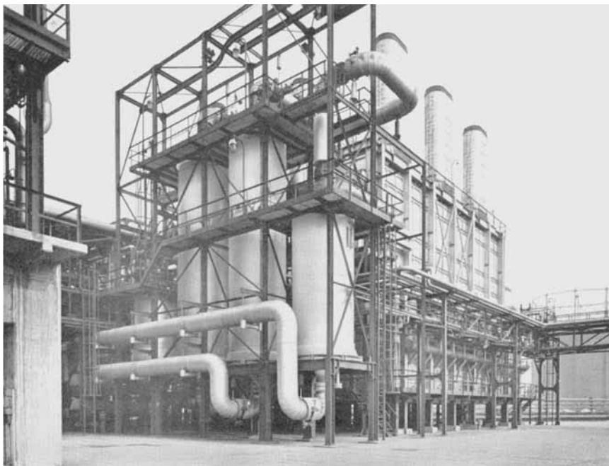
One of the three Platforming units at the Gelsenberg Benzin AG refinery at Gelsenkirchen, West Germany. In addition to high-octane motor fuel, high purity benzene is produced by separation from the reformat in a UOP Udex unit.
