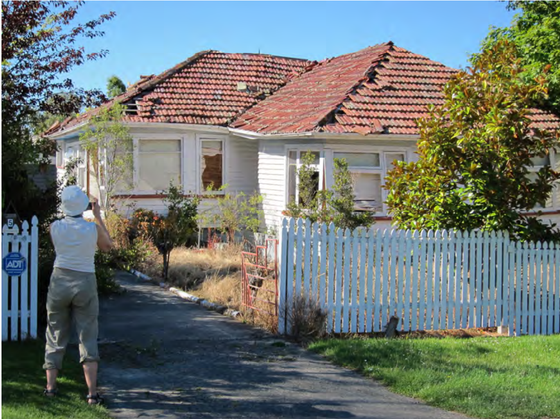
Damage from shaking to home in Hillsborough
