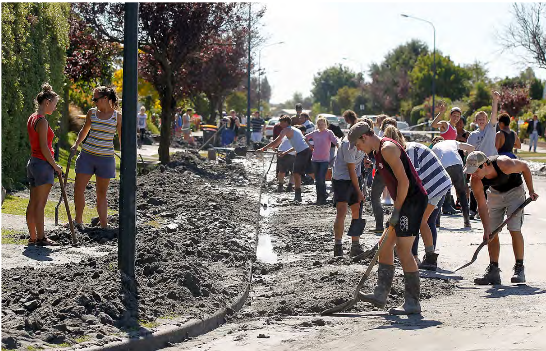
510,000 tones of mud and silt from liquefaction removed, much of it by an army of young volunteers
