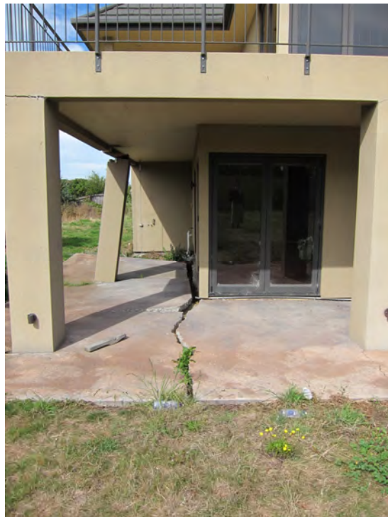
Liquefaction damage in Kaiapoi
