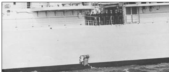
The patched bomb hole damage to GLASGOW at the waterline. Fortunately the bomb did not explode but damaged enough internal systems that reduced her ability to provide air defence to the Task Force. (RN)
