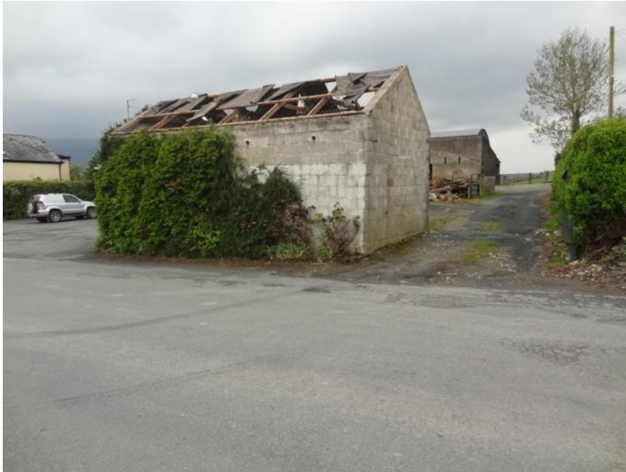
March 2013 – an old structure beside Carr’s shop due for demolition, the owners said it was a great incentive to do this to coincide with The Pure Mile
