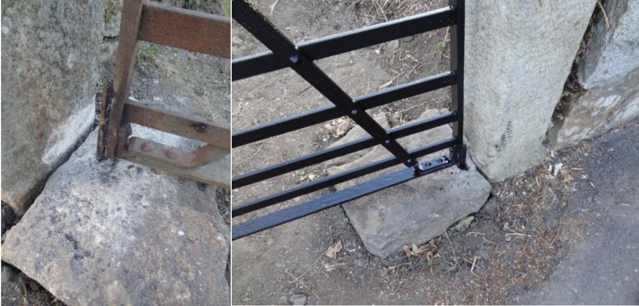
July 2013 – New ‘spud’ stones and welding on the base of each gates which sees them functioning again after over 30 years.
