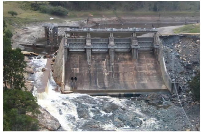
Photograph 3: Oaky River Dam Post-failure February 2013
