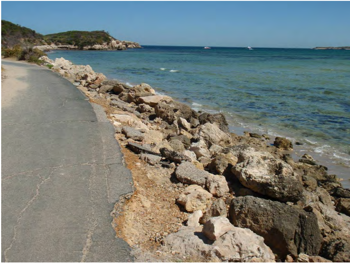
Figure 3: The seawall alongside the dual-use path (27/2/2009)
