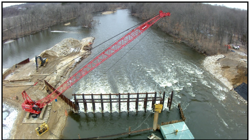
Crews remove the temporary water control structure at the former Otsego Township Dam.
