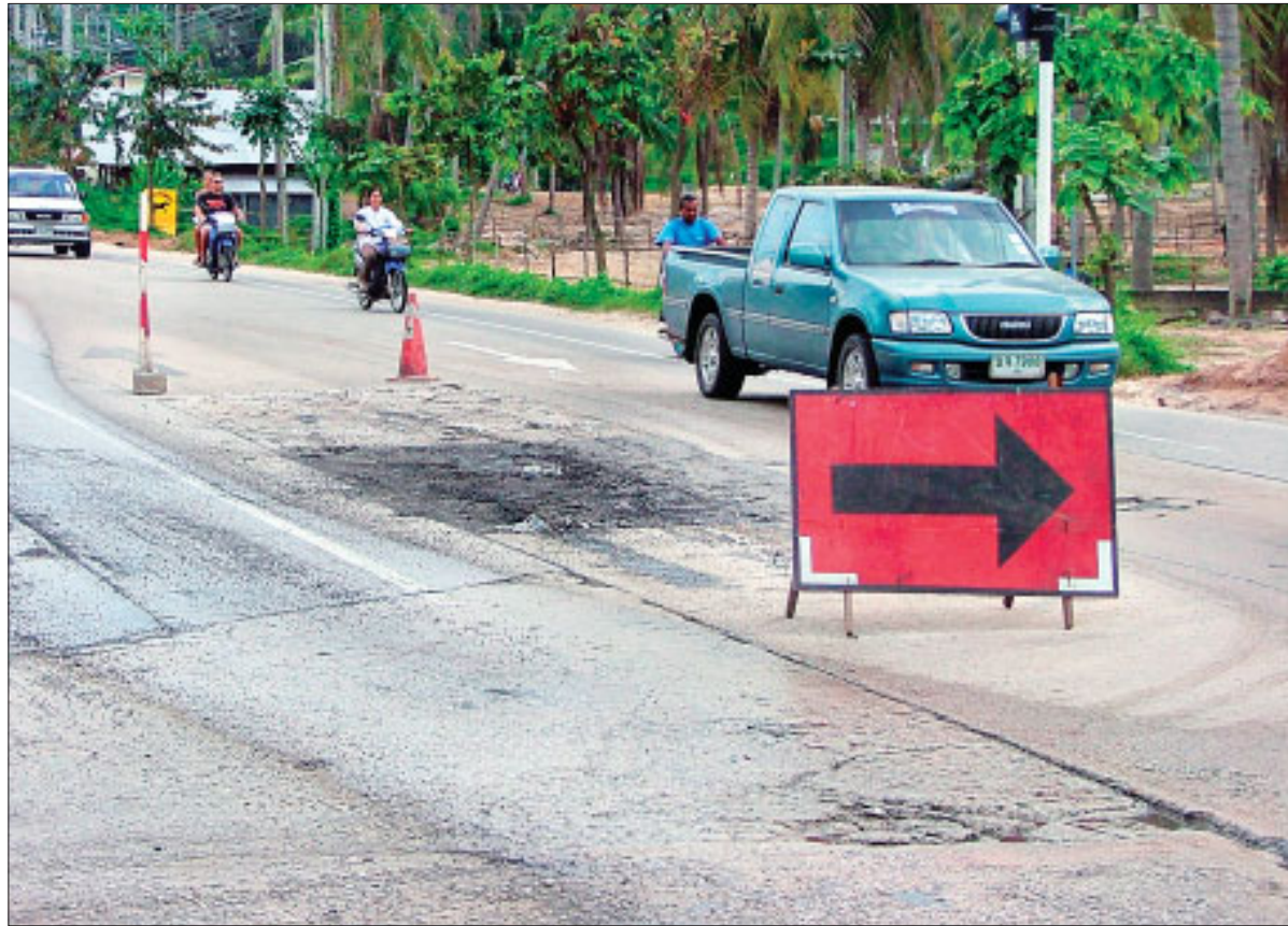
ROAD TO RUIN: People on Samui are angry at the lack of action to repair flood-damaged roads.
