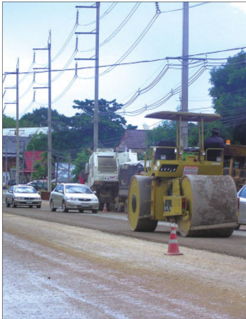
The work is part of a project to resurface Chao Fa West and Viset Rds all the way to Rawai Beach.
