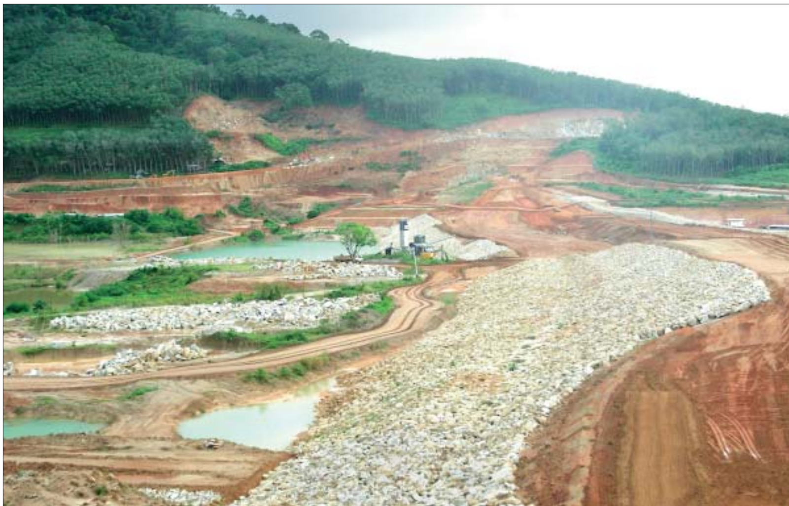
The earthen dam that will create the island's second reservoir at Bang Neaw Dum in tambon Srisoothorn, Thalang, is now about 75% complete. The Irrigation Department hopes the reservoir will be ready to supply water by next June.
