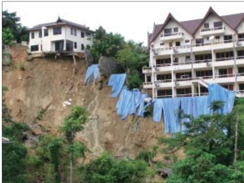
The landslide left the foundations of homes and a large apartment block exposed.
