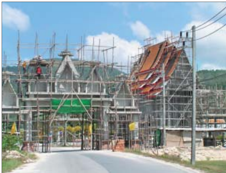
Workmen hang in the scaffolding over the incomplete gate while the roof is being added to the ordination hall at Wat Luangphu Supha.
