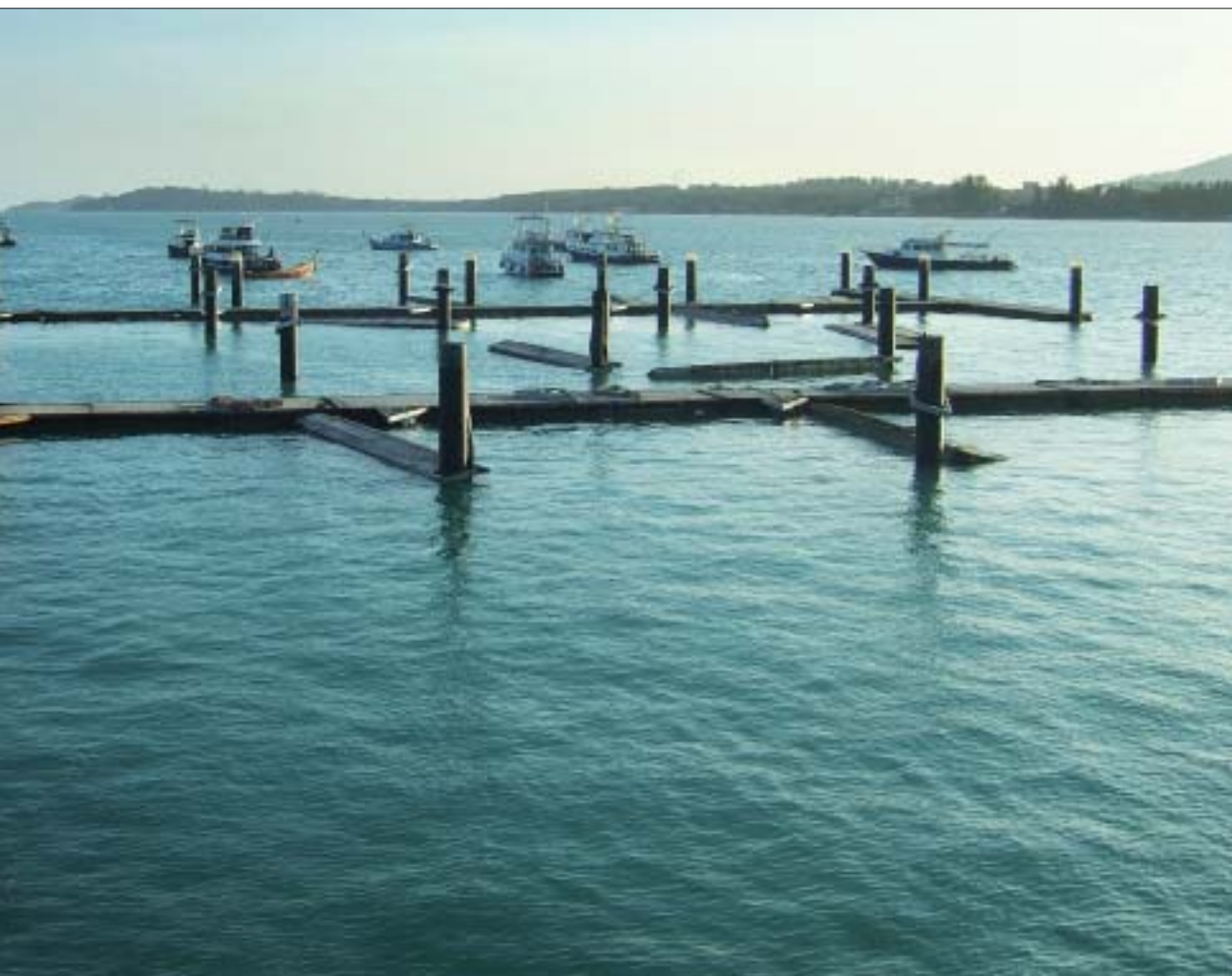
The southwest side of the 44-berth Chalong Marina project's Phase 1, as viewed from Chalong Pier. Scheduled for completion last September, Phase 1 is still not yet ready for visiting yachts. Phase 2, if built, would include a breakwater around the marina and expand the number of berths to 100.
