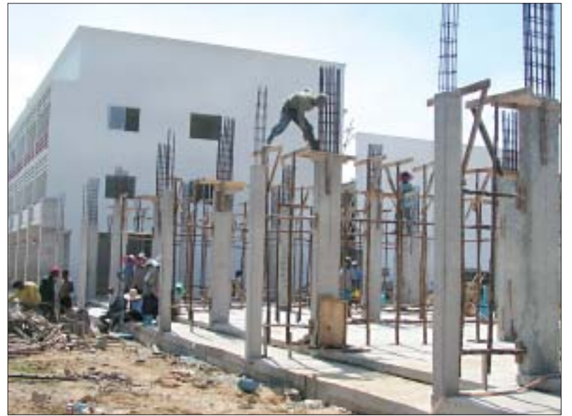
Work continues at the Top Land project on Wiset Rd, where all the commercial units have sold out.
