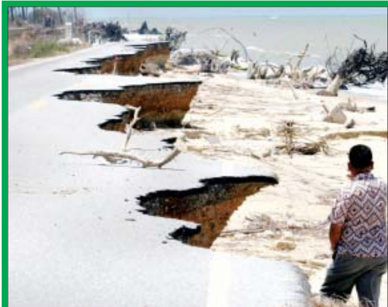
About one kilometer of the coastal road between Panarae and Yaring in Pattani province was badly eroded following heavy storm waves that coincided with high-tide conditions in the Gulf of Thailand. To travel between the two towns, local residents were forced to take alternative routes through "red areas" where insurgent activity is high.
