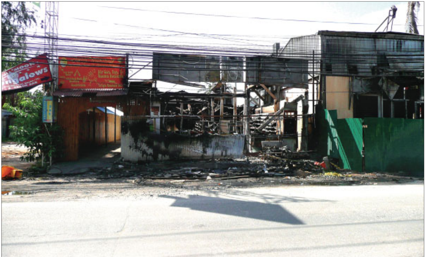
A 7-Eleven shop and a branch of the Bangkok Bank were incinerated in the fire that followed the truck crash.
