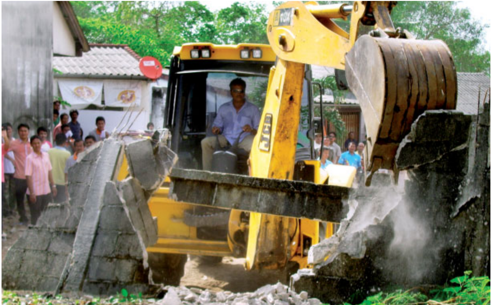
A backhoe destroys houses which were holding up construction of the new Phuket road. Meanwhile, local residents look on.
