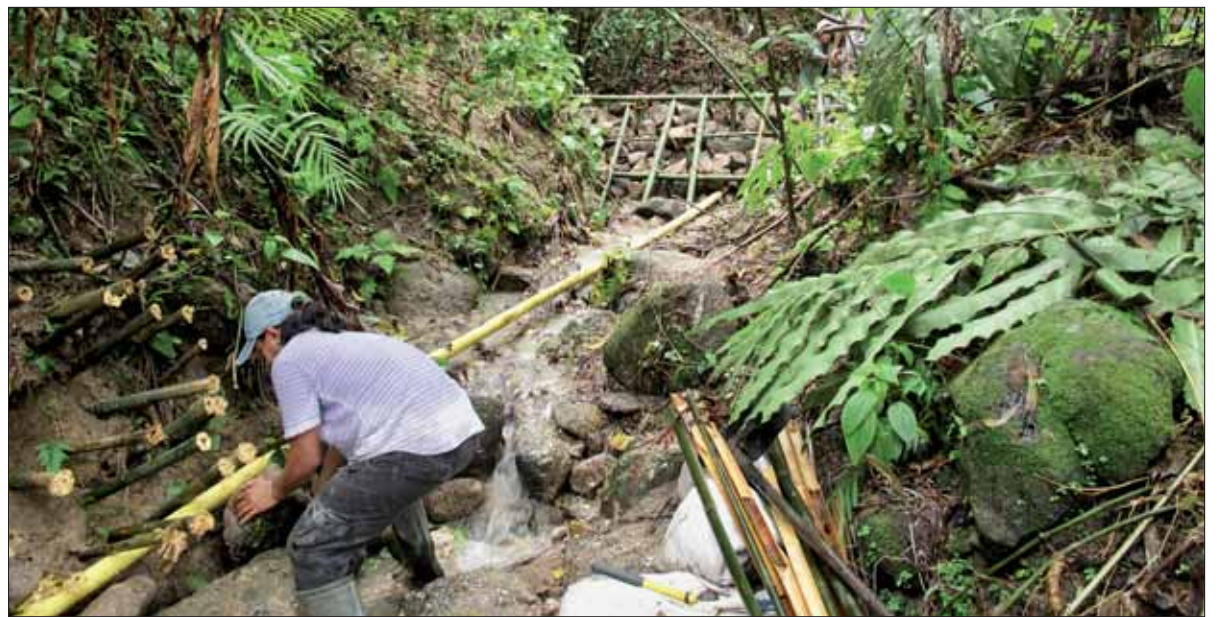
NATURAL SOLUTION: An army engineer installs piping at the site in the Kathu hills. Photo: Janpen Upatising
