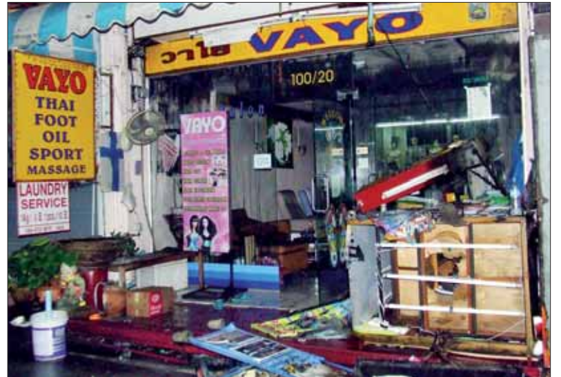
One of the neighboring shops also damaged by the fire. Photo: Atchaa Khamlo in the blaze.
