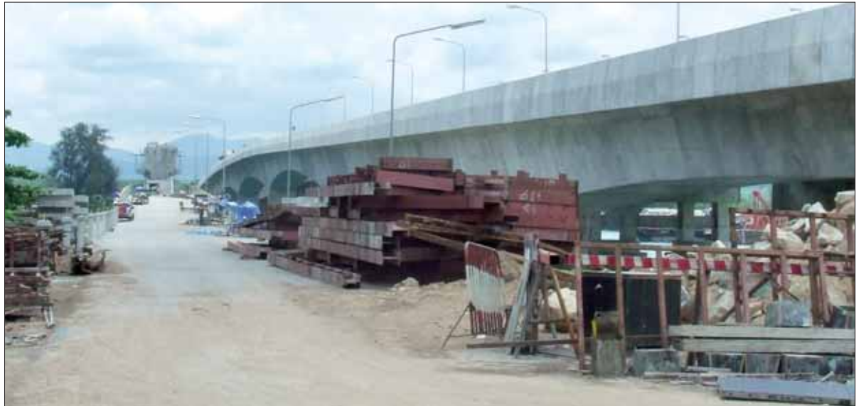
Construction will continue after the northbound lanes heading off the island open. Photo: Atchaa Khamlo
