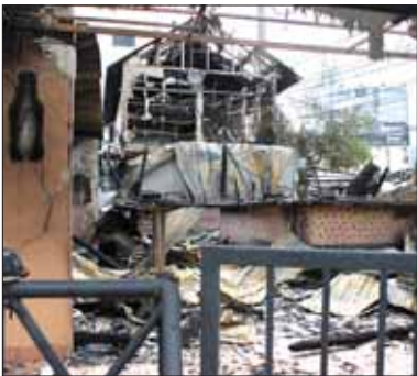
The remains of Kamala Beer Garden after the fire.
