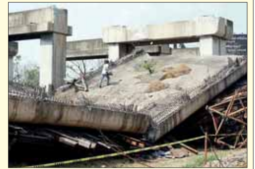
Collapsed Hopewell project. Photo: The Nation
