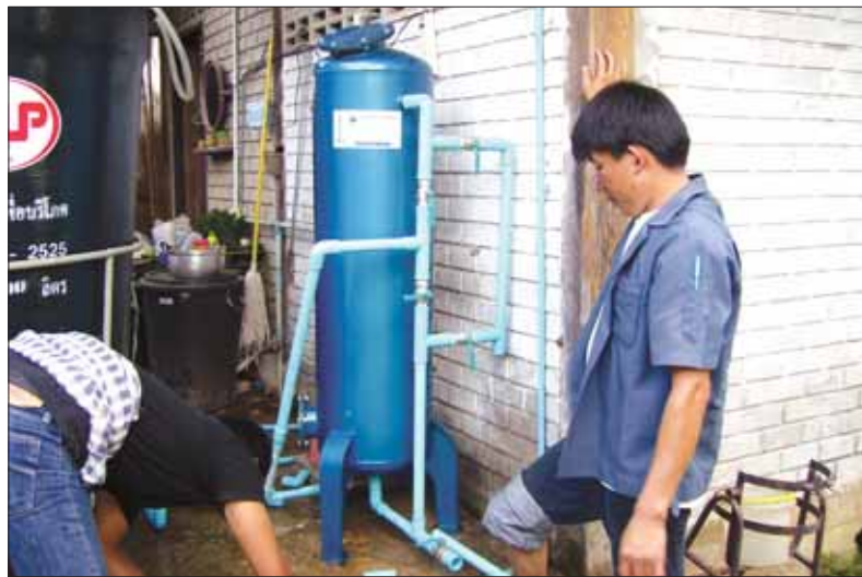
THAI STYLE PLUMBING: A Water Utilities management plan is strongly considered when applying for a Land Subdivision Permit. Photo: Geoff B
