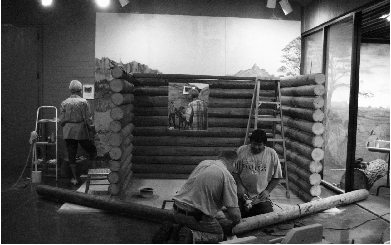
Construction of a cut-away miner's cabin in the Erickson Building as part of the "Gold Fever!" exhibit in 2007. Pictured (left to right) are Yvonne Ankele, Mary Ann Blomgren, Ron Van Gundy, and Tyler Mason.
