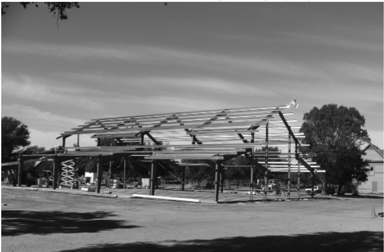
“Red barn” education support building construction, 2015. (Later dedicated as the Ledbetter Family Barn.)
