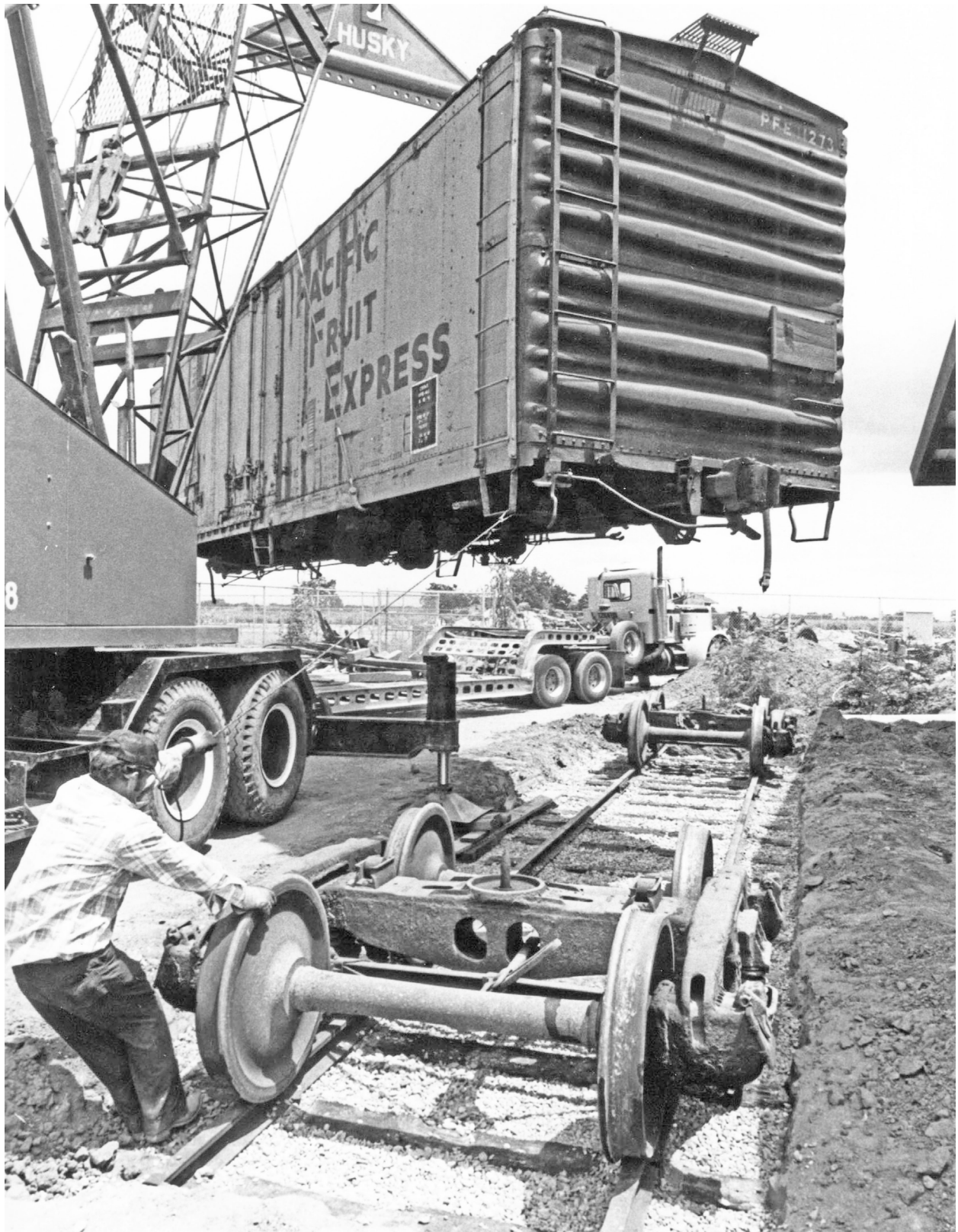
The Pacific Fruit Express ice car is lowered onto tracks north of the Tree and Vine Building in 1980. Built in 1957, the car is forty-five feet long and weighs 59,500 pounds. Ice was placed into ice bunkers at each end of the rail car. Fans mounted above the ice moved the air to keep produce and other goods cold.
