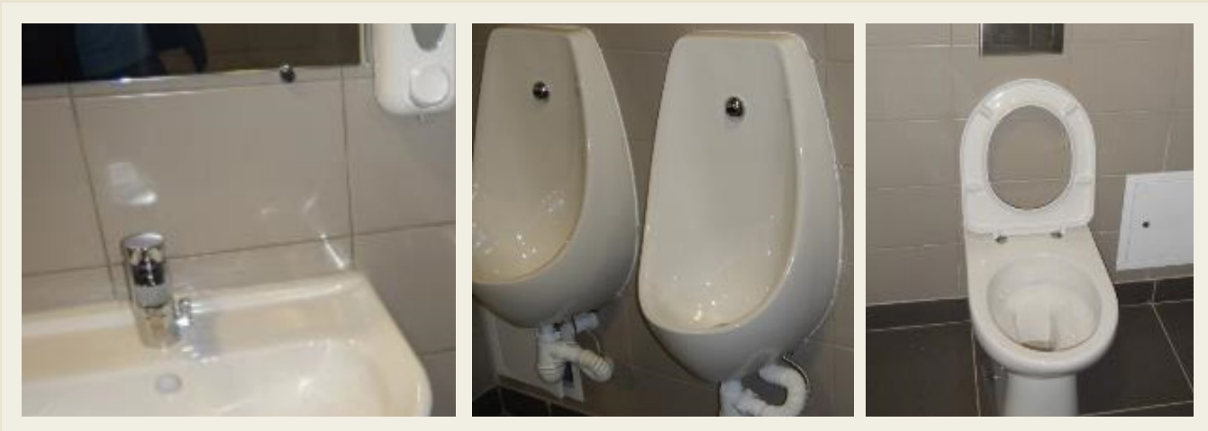
Fig. 28. Sanitary equipment of the stadium
