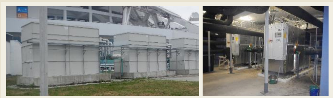
Fig. 49. Cooling towers and chillers at the stadium
