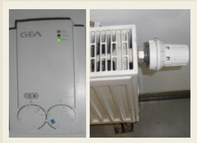
Fig. 46. 1: Fan coil control panel; 2: Radiator with a thermostatic valve
