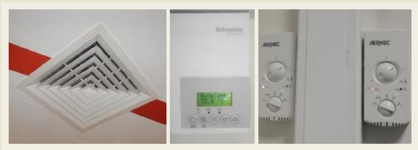
Fig. 3. Fan coils with control panels
