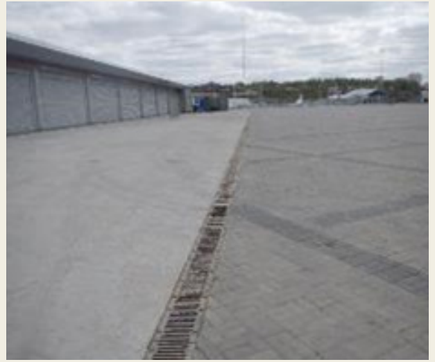
Fig. 43. Elements of the drainage system at the stadium
