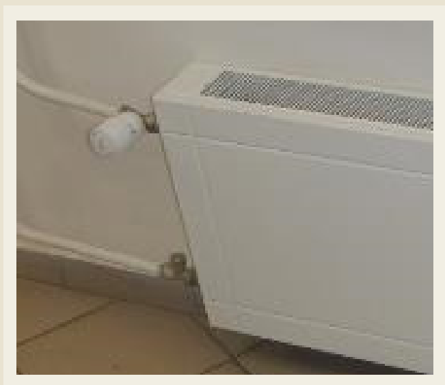
Fig. 4. Radiator with a thermostatic valve
