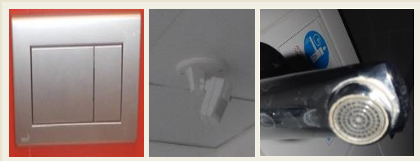
Fig.13. The stadium's water-saving equipment.
