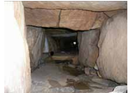
Figure 45 Structure of stone culvert below road surface Photo: Simon Wiltshier, Hughes Trueman Pty Ltd 12 September 2007
