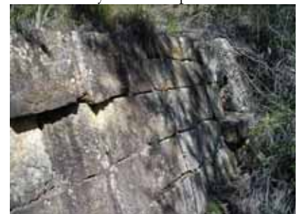
Figure 46 North face of culvert 6 Photo: Simon Wiltshier, Hughes Trueman Pty Ltd 12 September 2007
