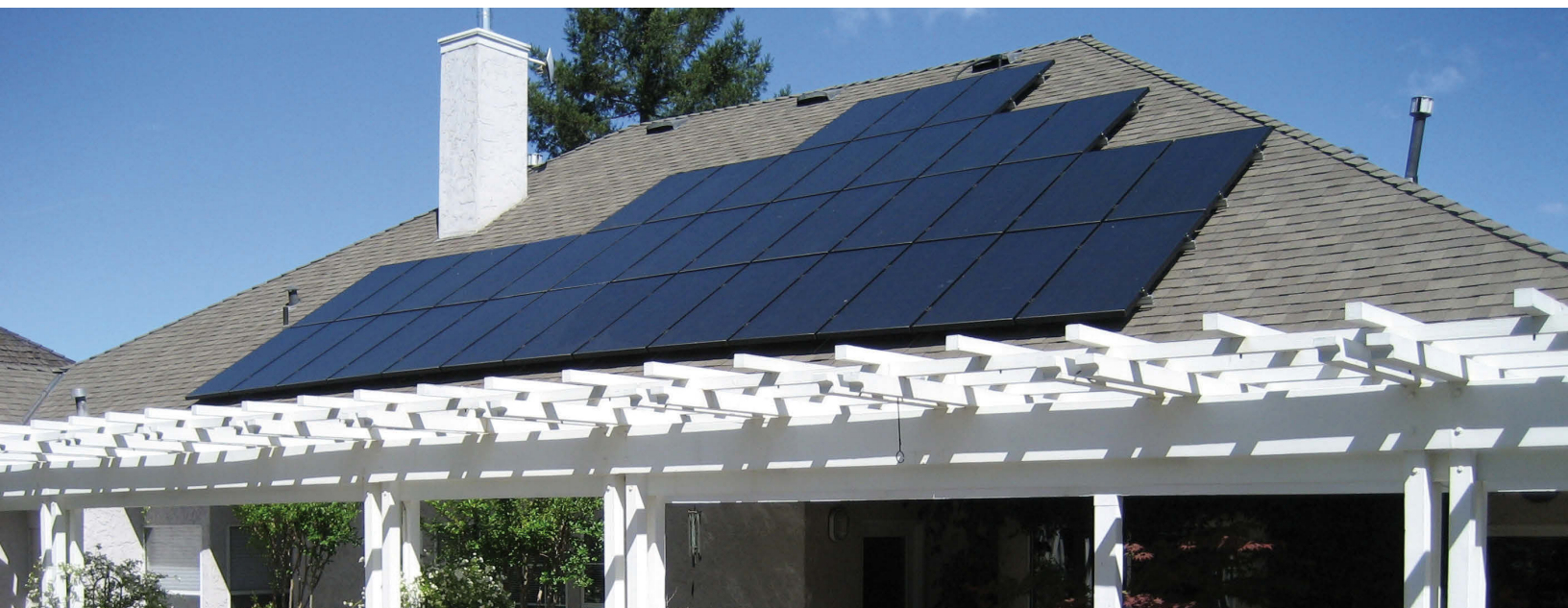
Residential PV installation in California
