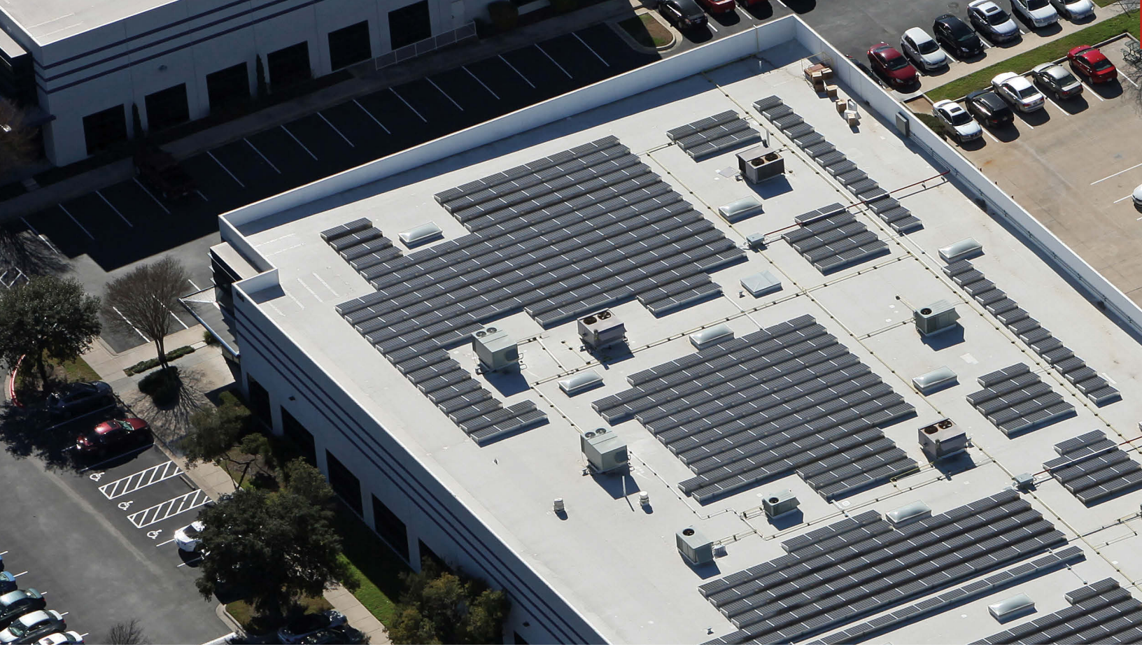
Commercial PV installation in Austin, Texas
