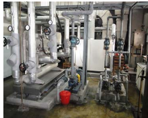
[Photo20] Air Conditioning Facilities (Chiller)
