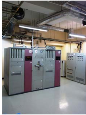
[Photo26] 2kW VHF TV Transmitters
