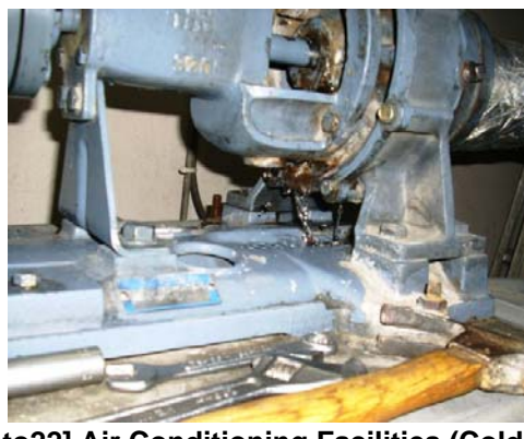
[Photo22] Air Conditioning Facilities (Cold water pump) corroding due to water leakage.
