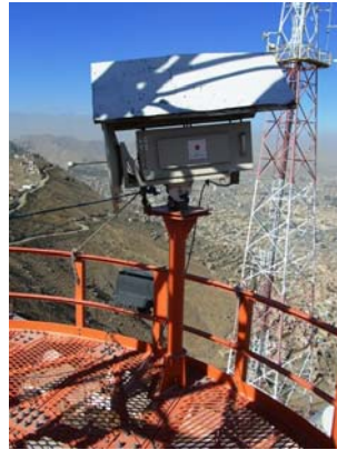
[Photo30] FPU receiving antenna
