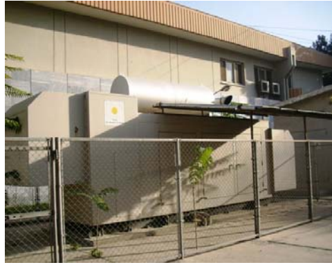
[Photo18] Power Supply System for Emergency
