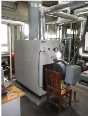
[Photo21] Air Conditioning Facilities (Boiler)
