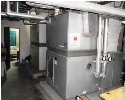
[Photo19] Air Conditioning Facilities (AHU)
