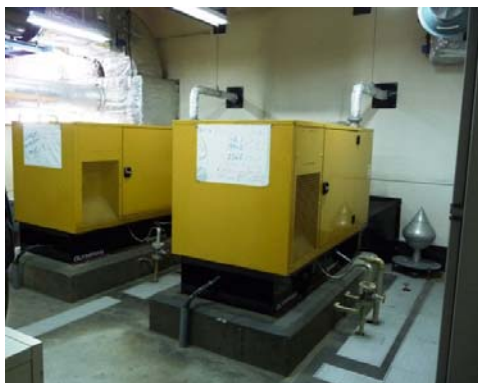
[Photo31] Generator for Emergency
