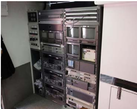
[Photo13] System Rack in OB Van
