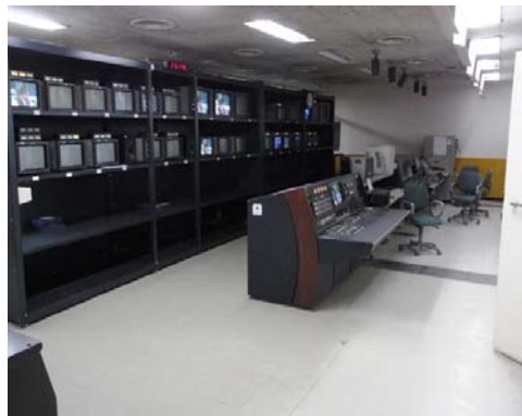
[Photo2] Master Control Room
