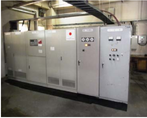
[Photo17] Low Voltage Power Distribution System (Right one is replacement of AVR installed by RTA)
