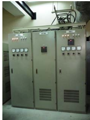
[Photo32] Low Voltage Power Distribution System
