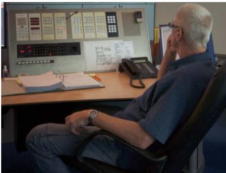
Figuur 6.17: Centrale controlekamer
