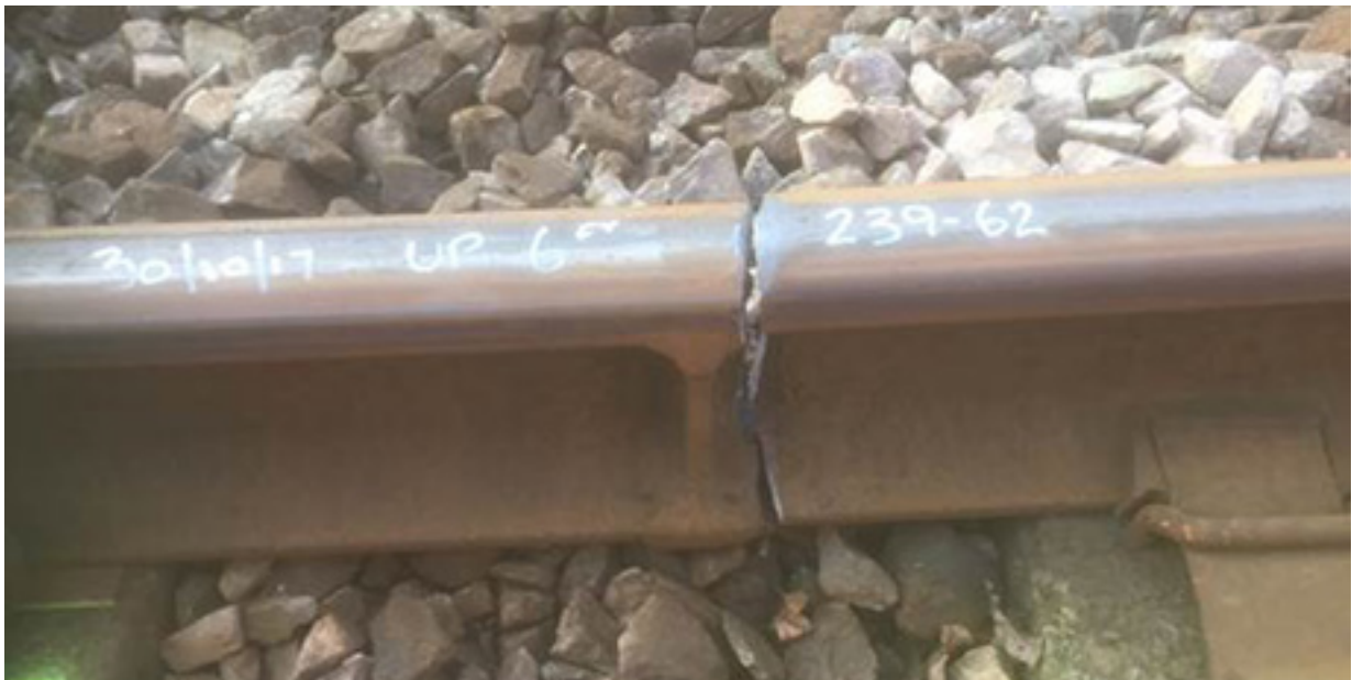
Figure 5: Broken weld 44.9 miles (72.2 km) from Robeston (courtesy Network Rail)
