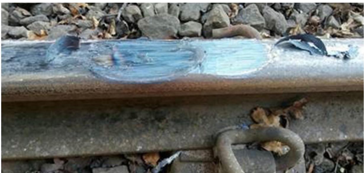
Figure 7: Damage to the rail head 67.2 miles (108.1 km) from Robeston (courtesy Network Rail)
