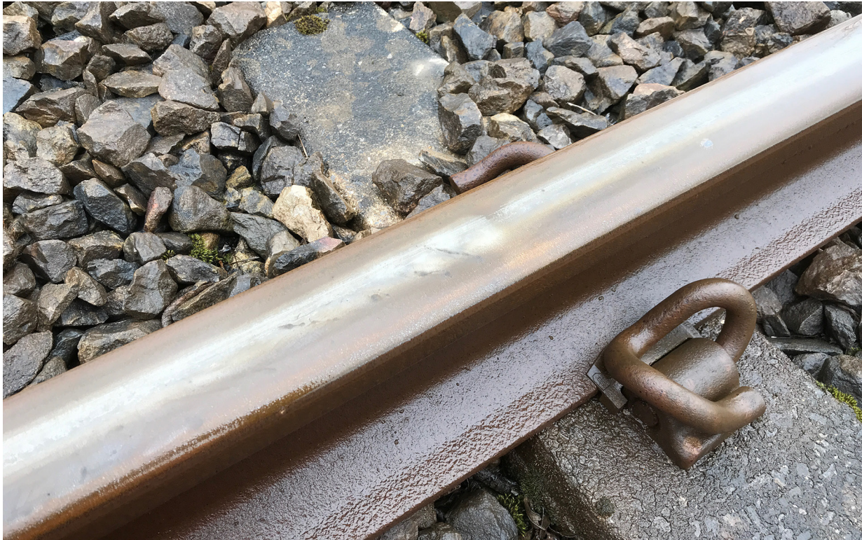
Figure 4: Rail head damage (six foot rail) 43.2 miles (69.5 km) from Robeston, still visible in April 2018
