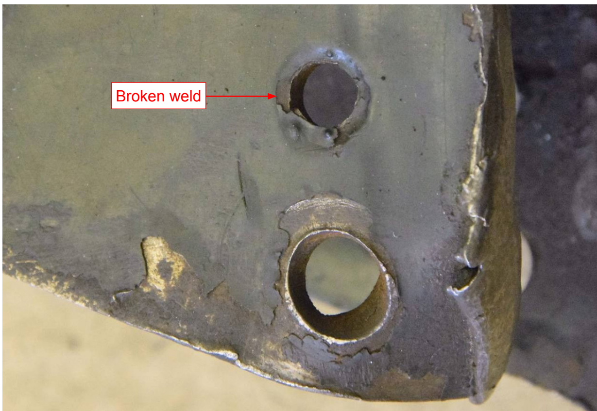
Figure 16: Inside corner of block holder from wheel position 5 (courtesy Serco Rail Technical Services)
