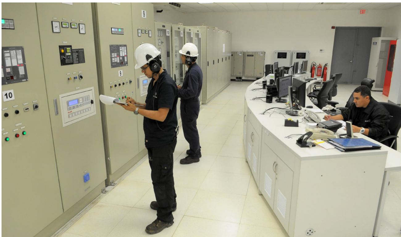
Operators of the two-stroke units at Miraflores Power Generation Plant
