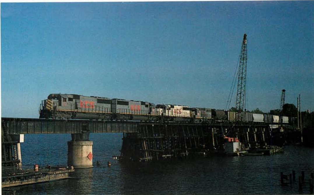
Two Kansas City Southern SD60s lead train 5 southbound over new bridge construction near Mooringsport, La., just north of Shreveport. KCS, in the process of absorbing regional MidSouth, continues to be one of the West's most successful railroads, boasting a healthy first-quarter profit. John Gieske
