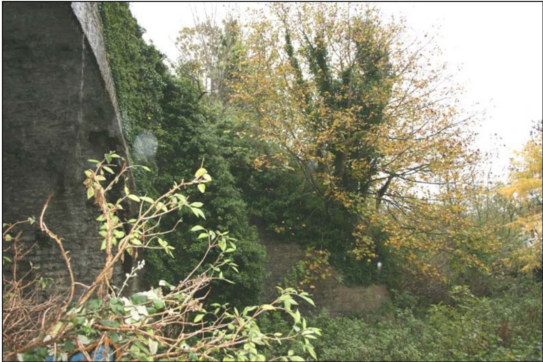
FHBS-11-BH-10 ~ South west buttress with tree and extensive vegetation rooted in masonry
