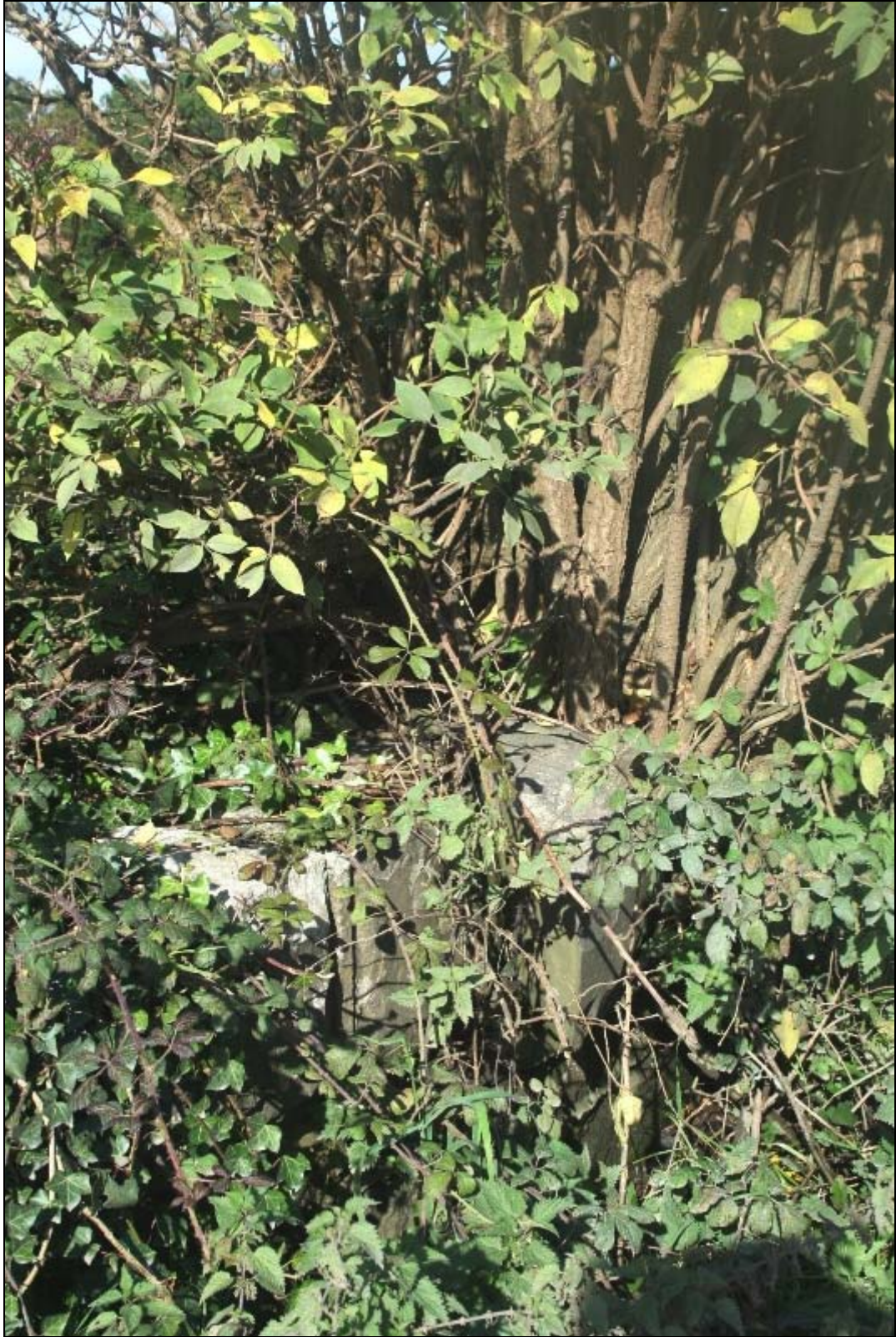
FHBS-12-BH-05 ~ Tree rooted on west parapet and dislodging stones
