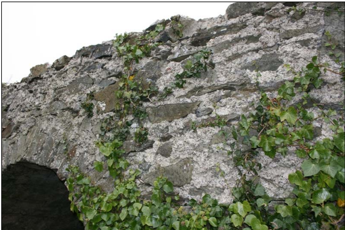
FHBS-10-BH-05 ~ Detail of stone and jointing mortar on exterior of south parapet
