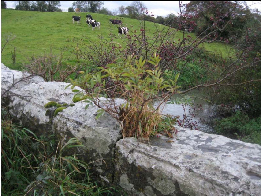
FHBS-12-NH-03 ~ Elder growing on downstream parapet wall
