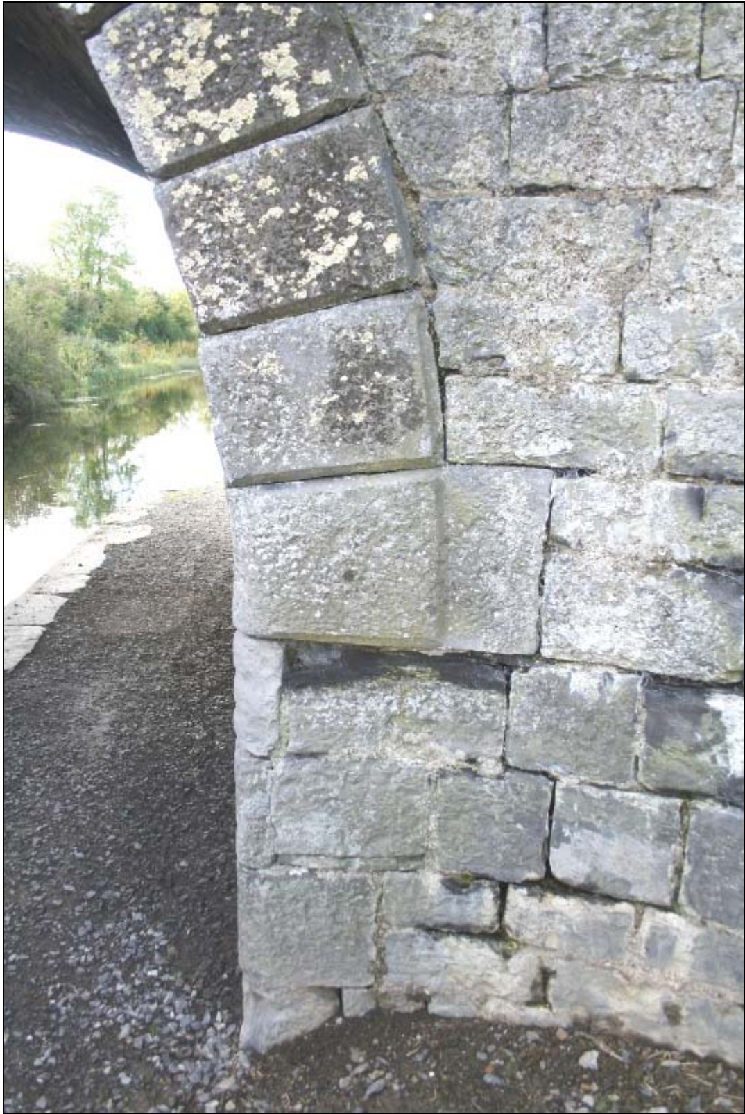
FHBS-15-BH-06 ~ Remains of lime render on north abutment of east side of canal bridge
