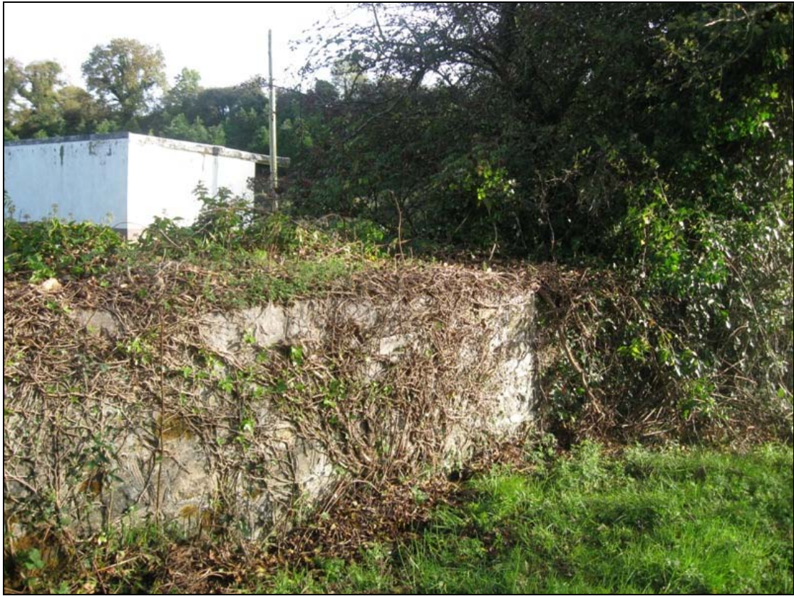
FHBS-02-NH-01 ~ Ivy coverage on bridge parapet
