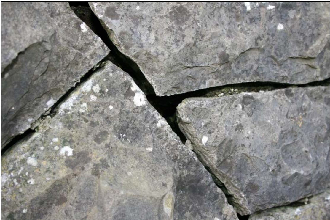
FHBS-03-NH-02 ~ Crevices in parapet wall
