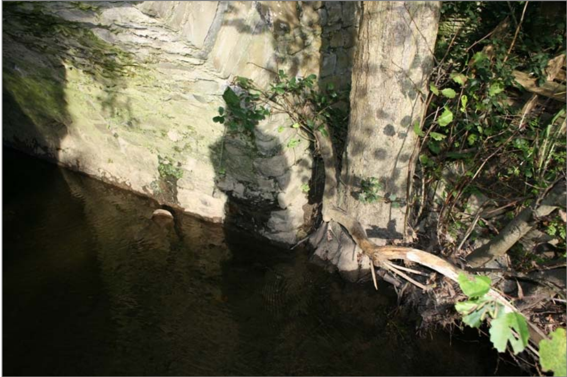
FHBS-01-BH-07 ~ Tree rooted underneath east elevation
