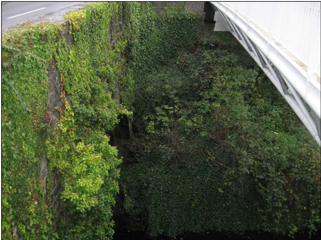
FHBS-13-NH-04 ~ Ivy on downstream parapet wall
