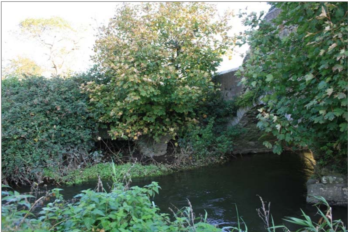
FHBS-01-BH-06 ~ Arches in boundary wall on north bank to western side of bridge
