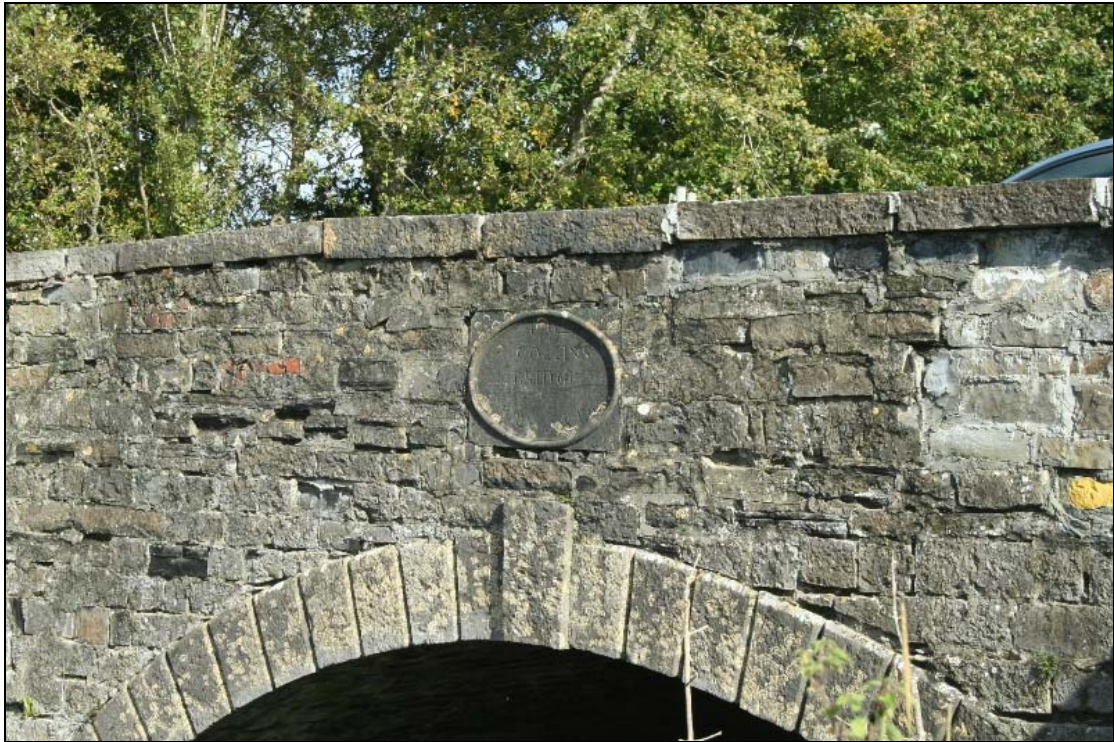
FHBS-15-BH-05 ~ Detail of name plaque and keystone on west elevation of canal bridge
