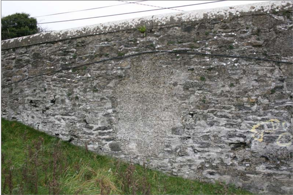
FHBS-07-BH-05 ~ Cast concrete repair on bulging section of southern abutment on eastern side of bridge
