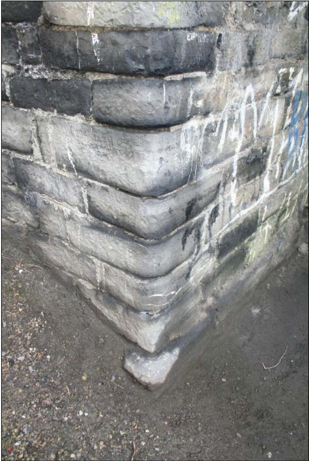
FHBS-14-BH-06 ~ Rounded arris to masonry beside towpath.
