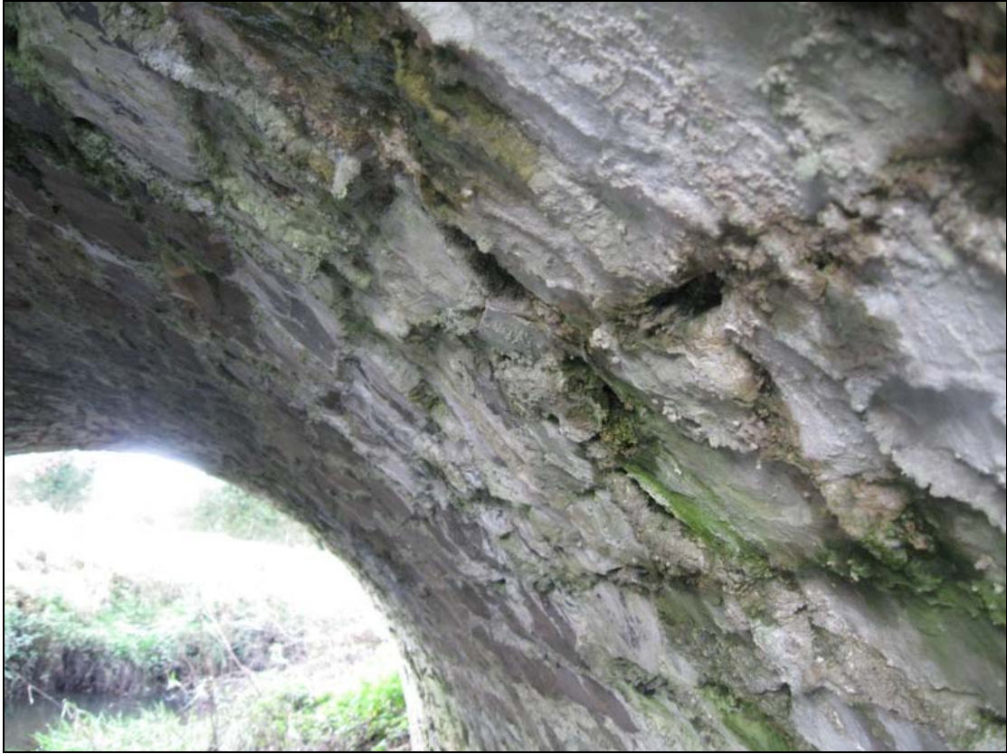
FHBS-03-NH-01 ~ Crevices on bridge – bat roosting potential
