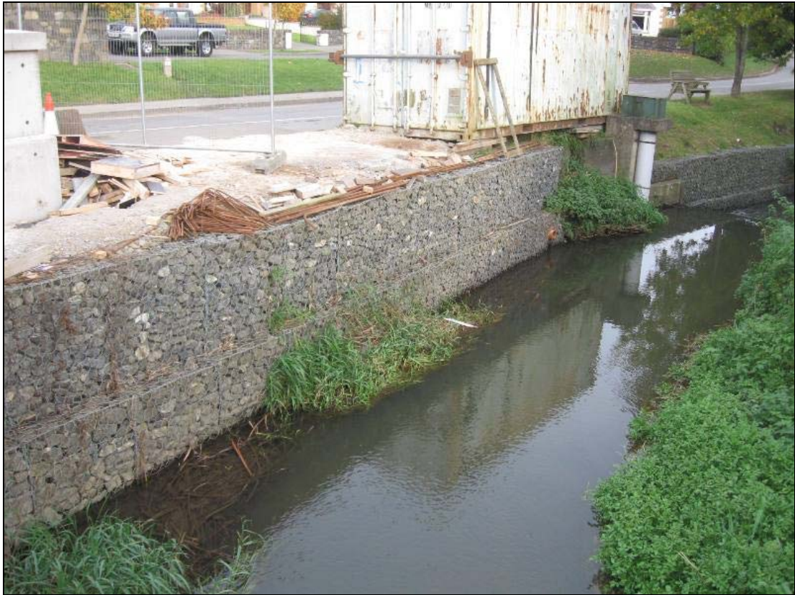
FHBS-06-NH-02 ~ Gabion structures on downstream bank
