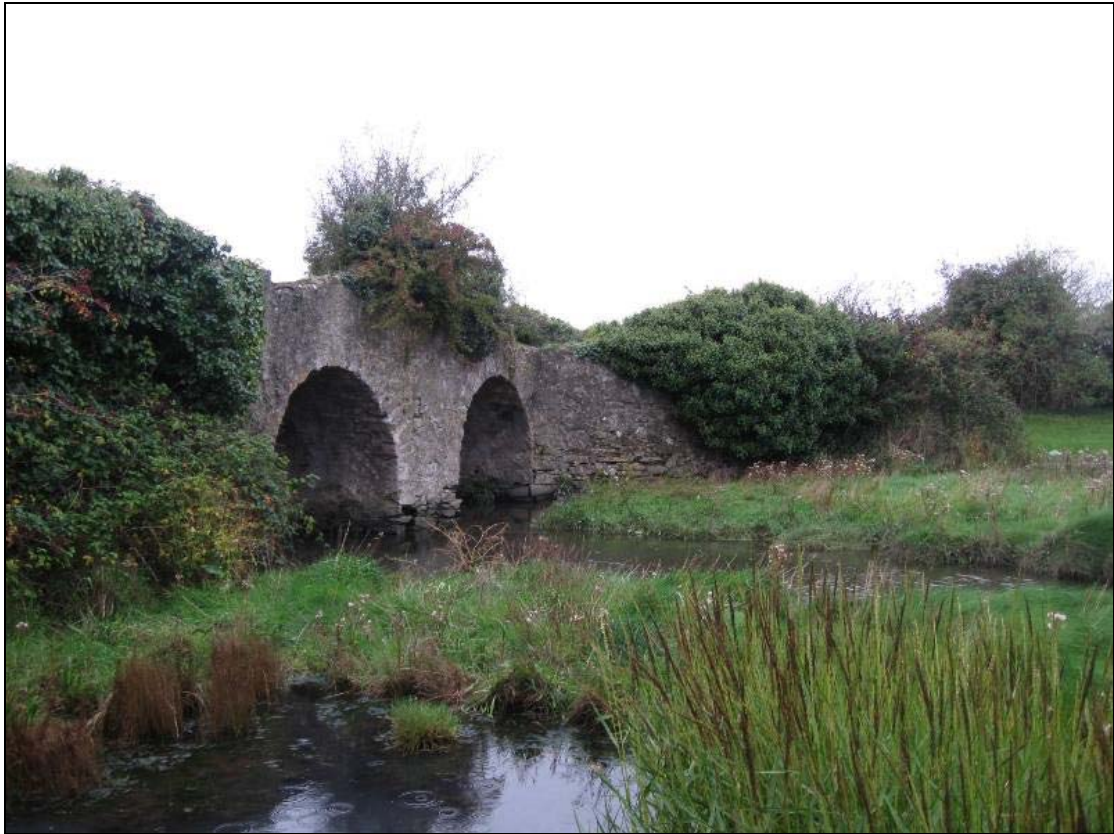
FHBS-10-NH-05 ~ Dense ivy on bridge sidewalls
