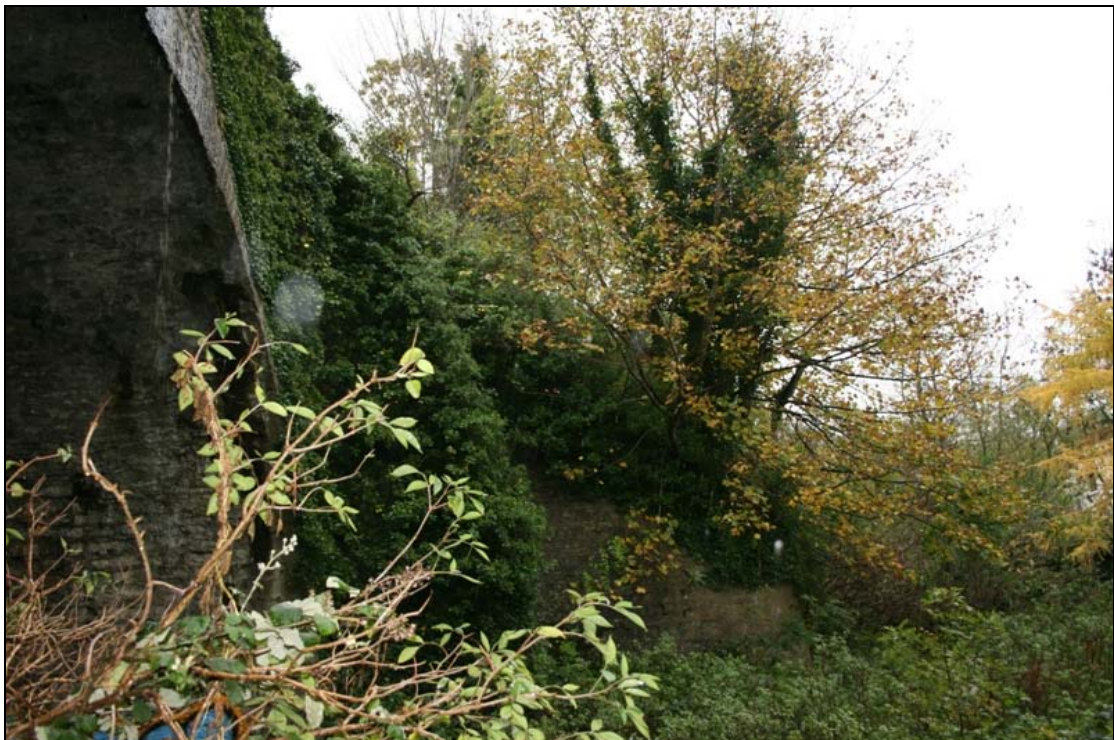
FHBS-11-NH-03 ~ Dense ivy growth on bridge buttress
