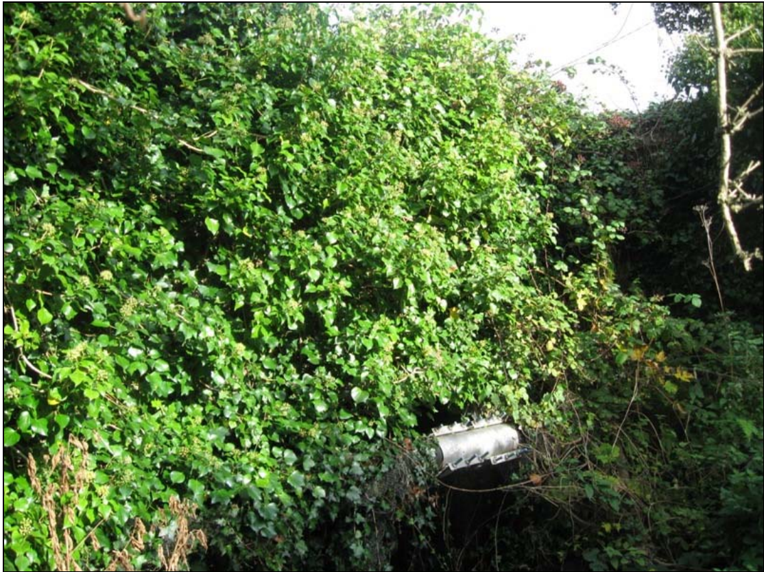
FHBS-05-NH-03 ~ Ivy on downstream parapet wall
