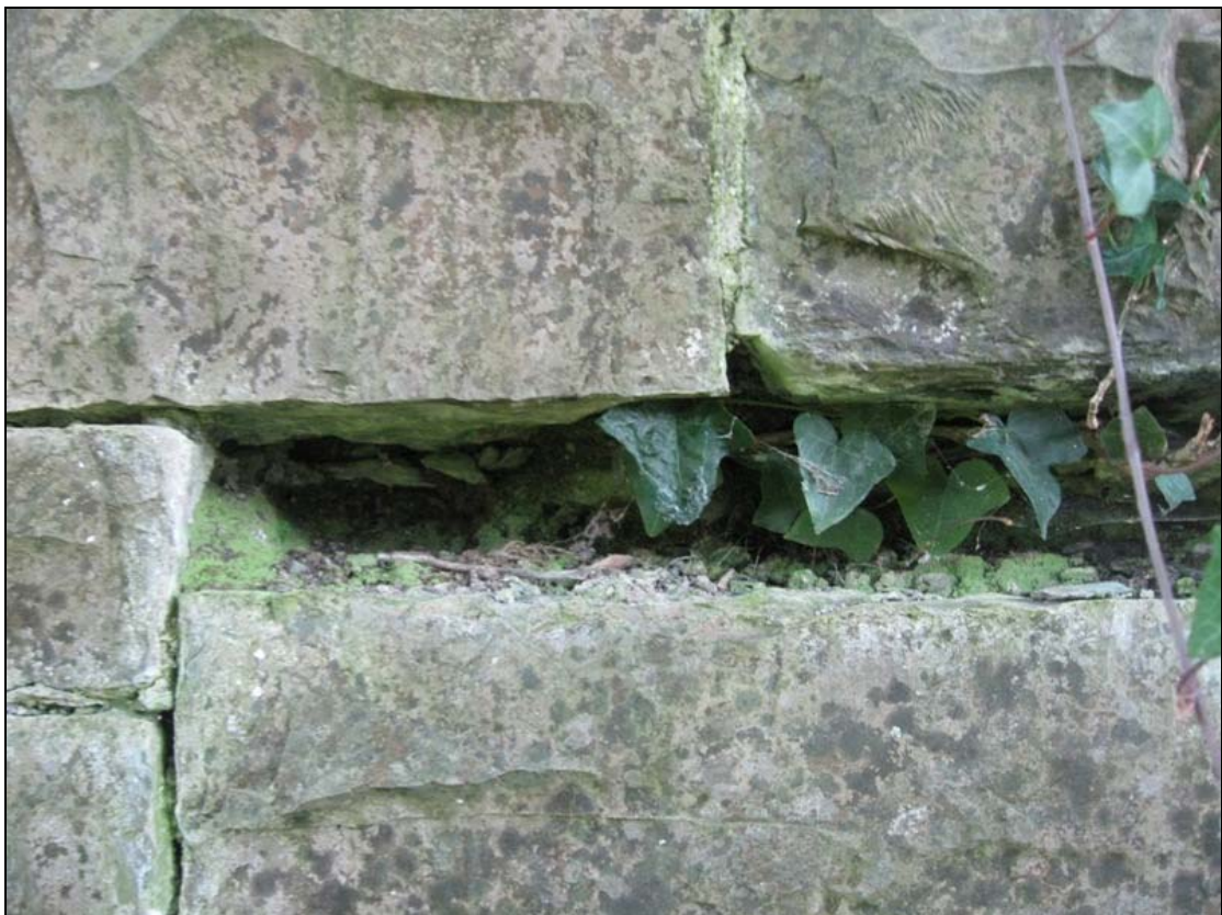
FHBS-04-NH-04 ~ Structural breakdown of parapet wall
