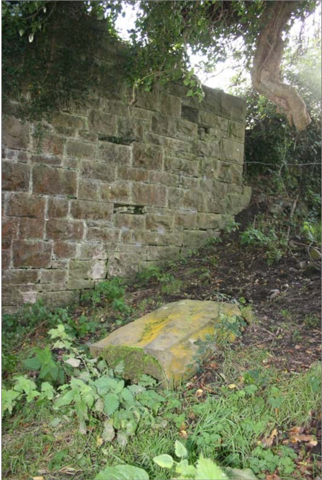
FHBS-04-BH-06 ~ Dislodged coping stone and stones missing from south abutment on west elevation.
