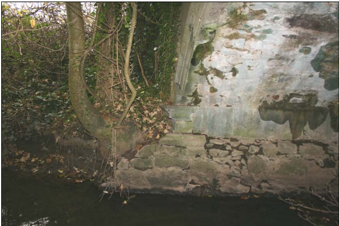
FHBS-09-BH-05 ~ Tree rooted on stone abutment on north bank of west side
