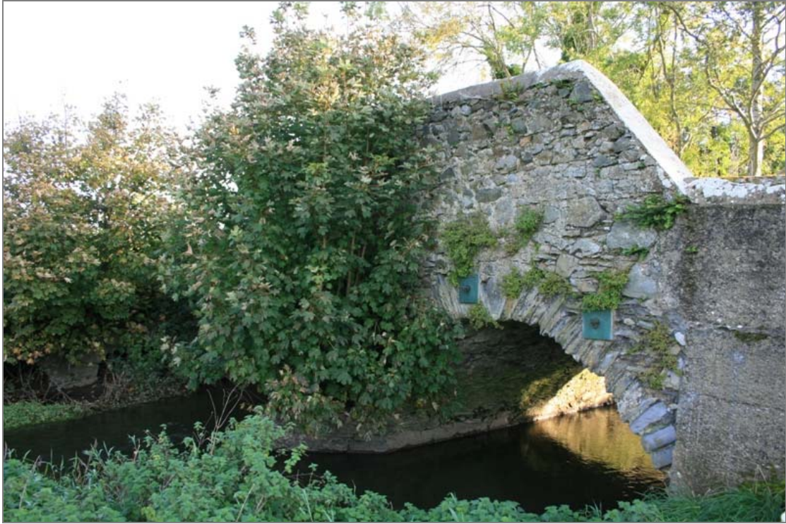
FHBS-01-BH-05 ~ Tree rooted on stone cutwater
