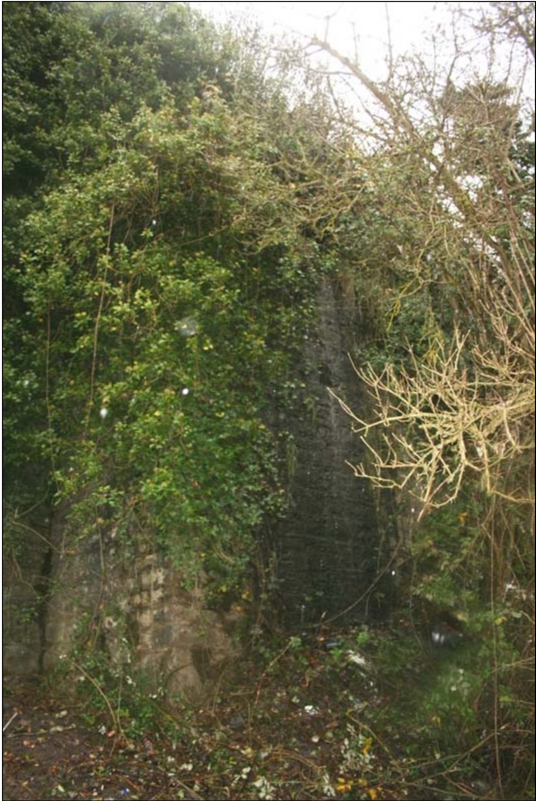
FHBS-11-BH-04 ~ North east buttress with road drainage washing over and vegetation rooted in masonry
