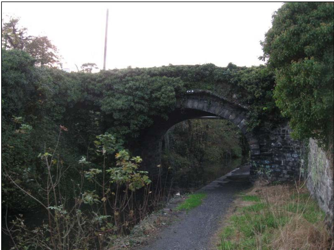
FHBS-14-NH-02 ~ Ivy coverage on bridge parapet wall
