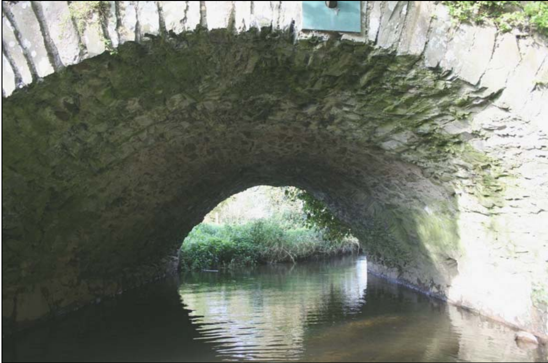
FHBS-01-NH-01 ~ Bridge underarch with crevices – Bat roosting potential
