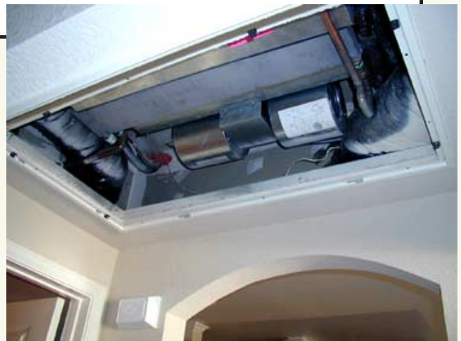
Pictured here: A fan coil unit installed.
