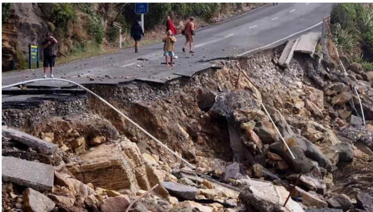
State Highway 6 near Punakaiki (on the West Coast) is severely damaged. [via Stuff.co.nz ]
