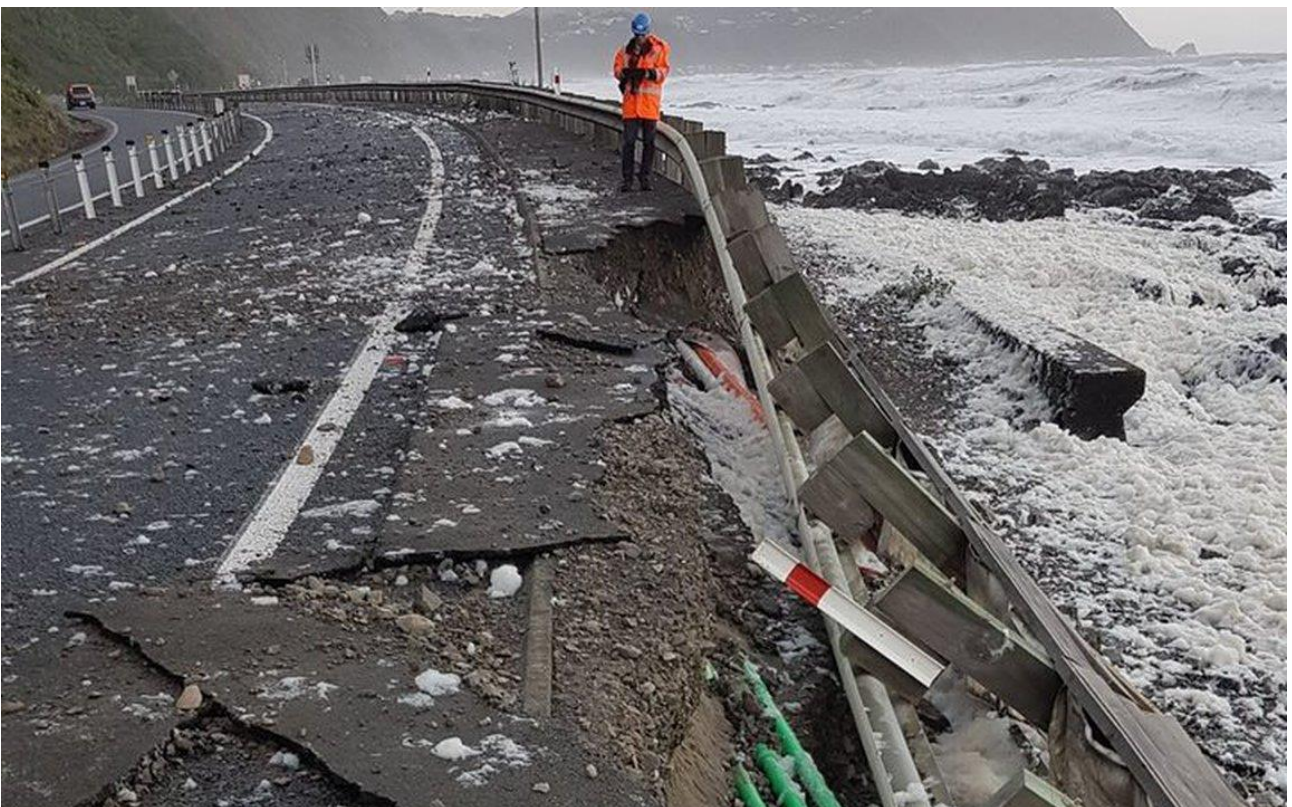
Damage to State Highway 1 north of Wellington. [via radionz.co.nz ]
