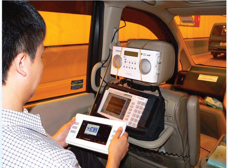
本署電子督察在第一期工程的每條隧道內量度數碼聲音廣播訊號。 Our electronics inspector measured DAB signals inside each tunnel of Phase I of the project.
