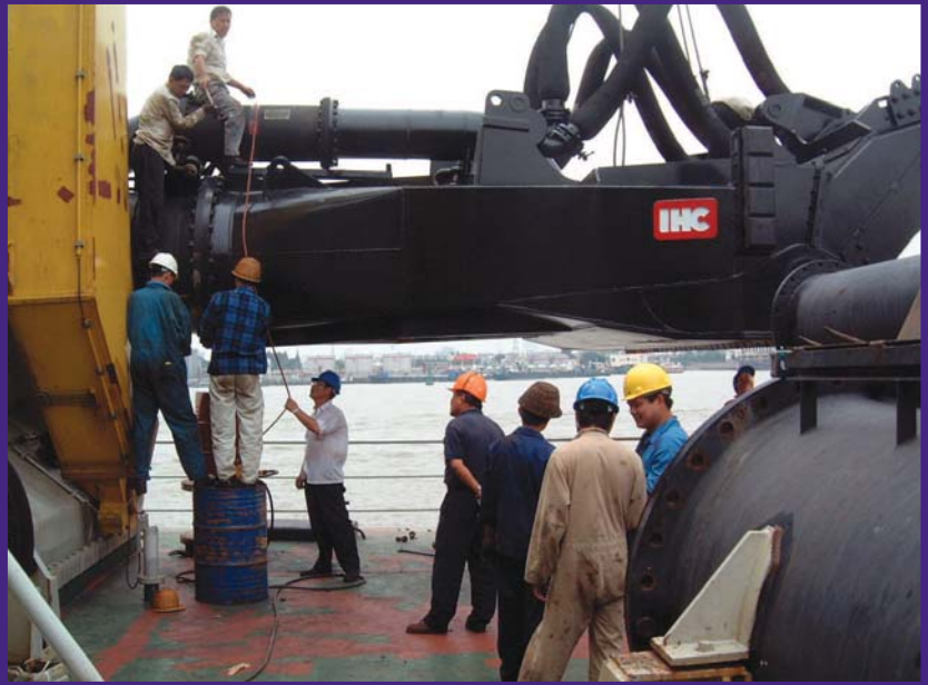
No shortage of hands: the SDC yard's crew mounting the 'Wild Dragon'® drag head to the XIN HAI LONG suction pipe
