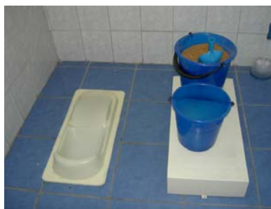
Figure 3. Interior of the double vault dry urine diverting toilet facility, built in conjunction with the school for 380 pupils: Hygienic, safe and easy accessible without leaving the school. (Source WECF)
