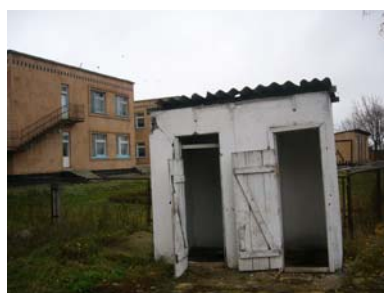
Figure 1. A latrine for 160 pupils, bad smelling and therefore far away from the school (source WECF)
