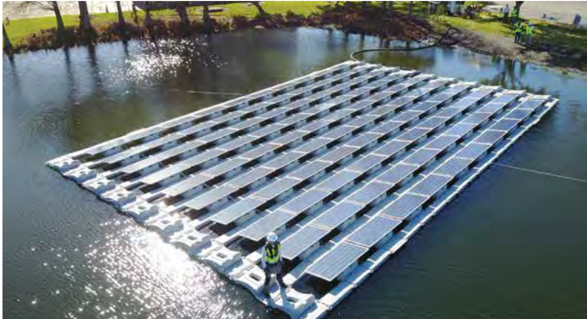
FIGURE 3.14. FPV project in Orlando, Florida, United States
