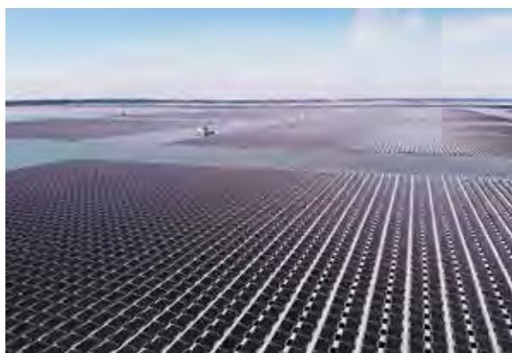
Source: © Sungrow. Note: kWp = kilowatt-peak; MWp = megawatt-peak.
