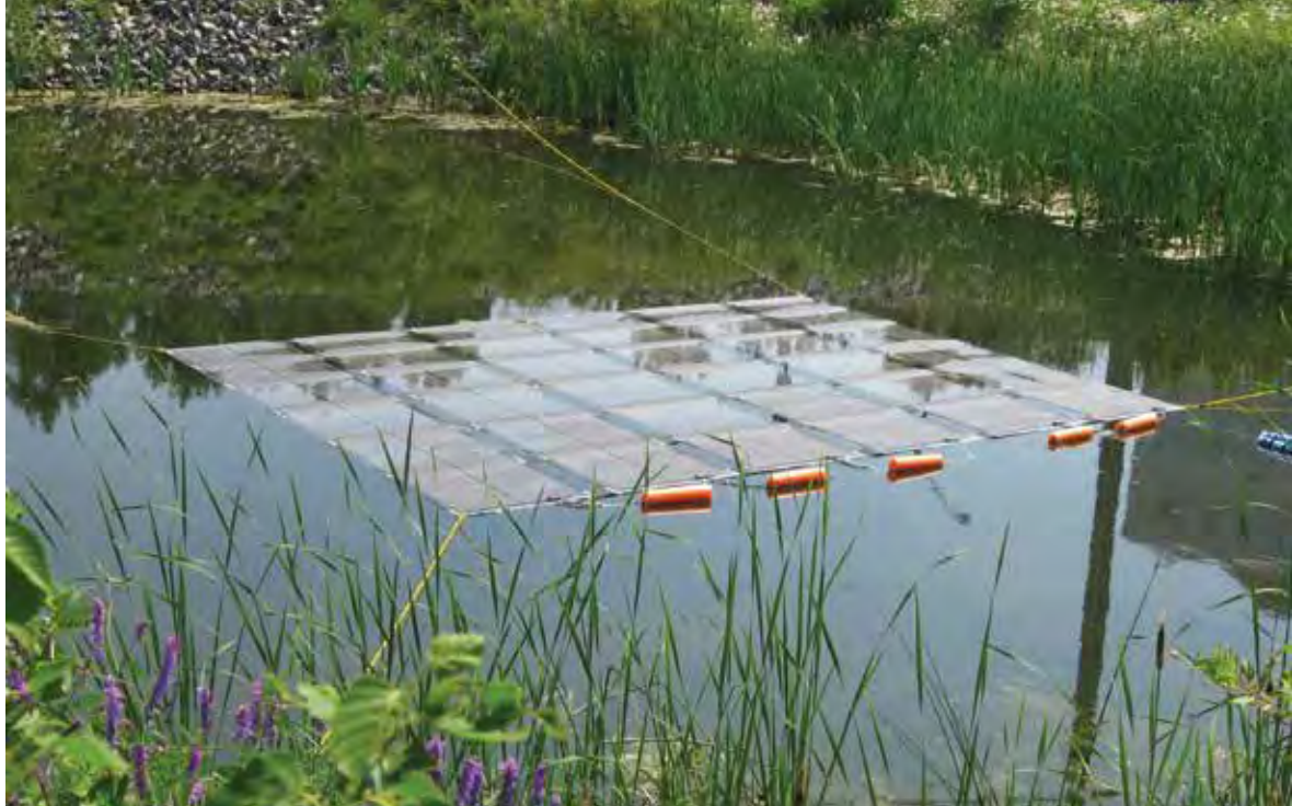
FIGURE 2.21. The 0.57 kWp MIRARCO Mining Innovation semi-submerged floating thin-film system in Sudbury, Canada
