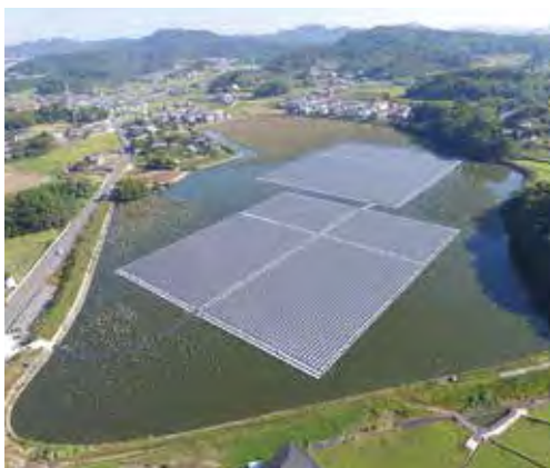
FIGURE 6.7. Examples of SMCC’s FPV systems in Japan
