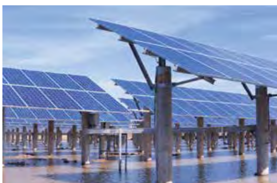
FIGURE 1.5. A “PV over water” installation
