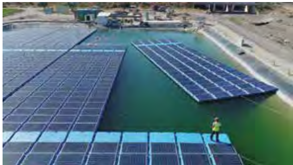
FIGURE 1.7. FPV system for covering of entire reservoir surface to reduce water evaporation
