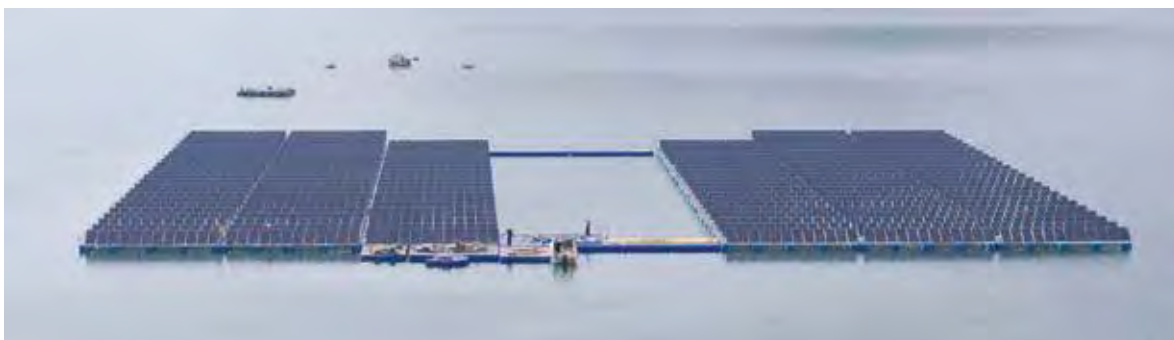
FIGURE 6.5. LSIS FPV installations in Korea
