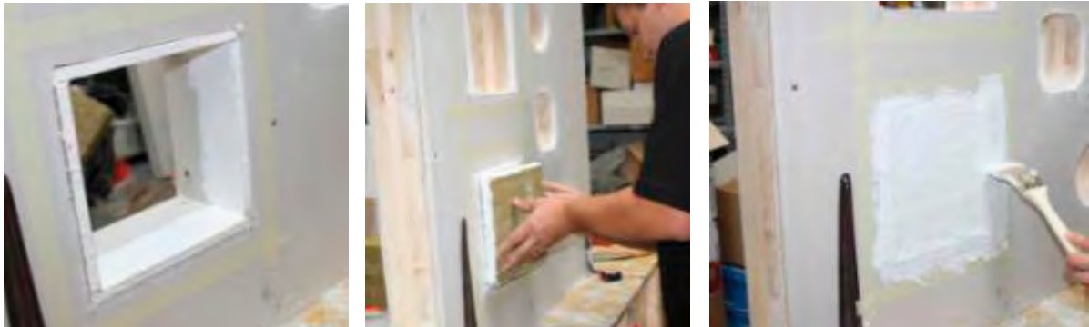
Figure 80: Installation of the soft partition in a sample body (left: reveal covering center: Installation of the mineral fiberboards that is coated on its edges, right: Overcoating of surface beyond the edge of 20 mm)
