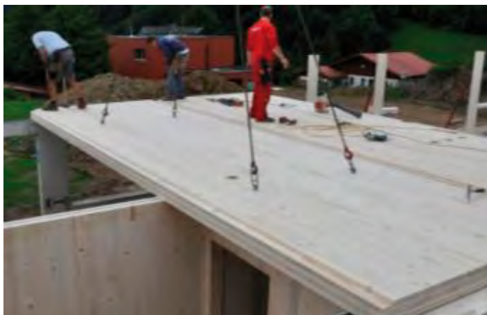
Figure 38: Continuous floors, if used with partition walls, need a suspension in order to prevent sound longitudinal conduction
