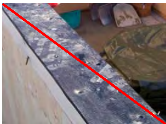
Figure 62: Inadmissible fastening of the elastic padding support using nails
