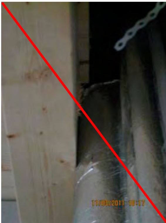
Figure 76: Due to a later extension of the shaft, non-combustible cladding of the wooden beam inside the shaft is not possible
