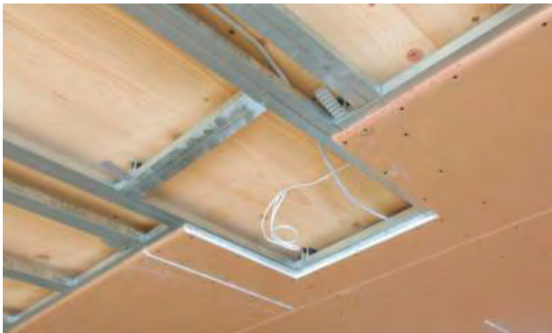
Figure 36: Floor system with whip arm and GKF with good sound protection properties, source: Knauf company
