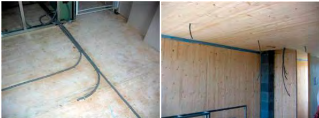
Figure 32: Laying of electric cables is to be executed in an airtight way for visible cross-laminated timber floors
