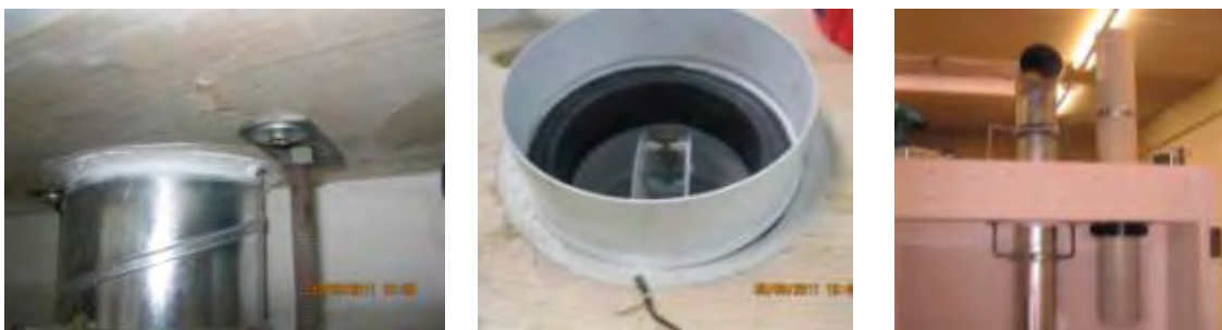
Figure 89: Rigid fastening of the ventilation pipe in the wood floor (left), fire protection closure based on intumescent materials with closing element FLI-VE (center), installation in sample body (right)
