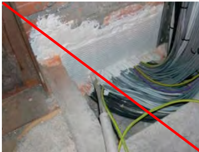
Figure 98: Cable bundle penetration with soft partition and too high configuration, source: Hilti company
