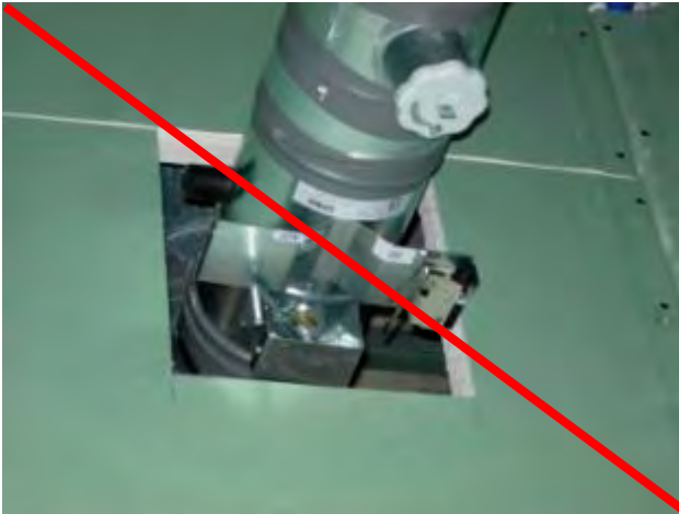
Figure 92: Installation of a fire protection flap in a unilaterally planked gypsum board stud shaft wall without partition (soft partition), source: Air Fire Tech company
