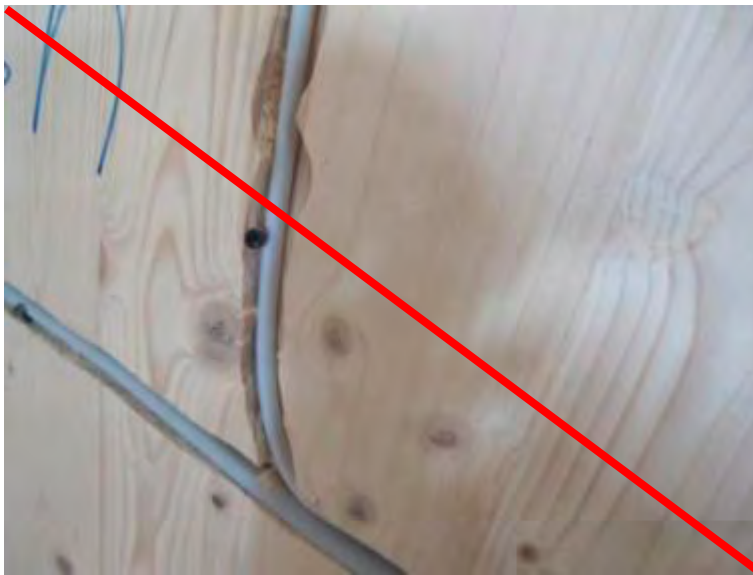
Figure 99: Direct installation of electric cables in cross-laminated timber is not recommended
