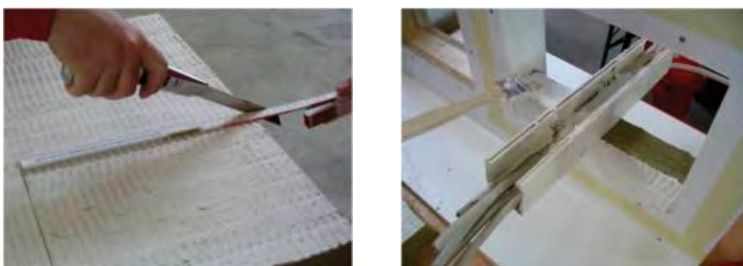
Figure 82: Cut to size of mineral fiberboard and coating of boards and reveal, source: Würth company
