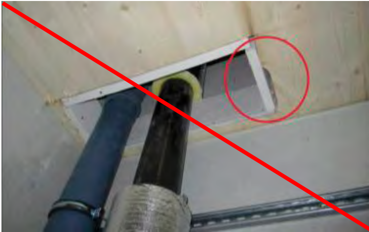
Figure 77: Installation of a reveal covering not over its entire surface
