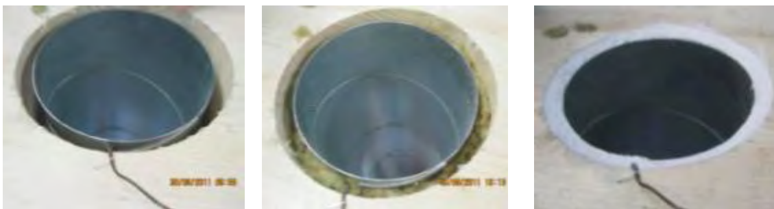
Figure 88: Insulation of the annular gap between ventilation pipe and wooden component with stone wool (center), application of an intumescent fire protection compound with a depth of about 15 mm (right)
