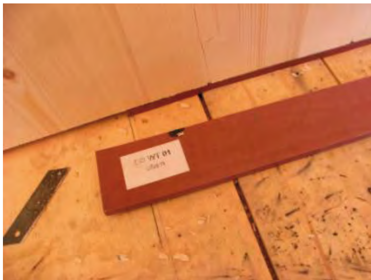
Figure 61: Sylomer supports in the padding support area for decoupling
