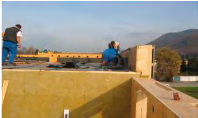
Figure 41: Vapor retarder (bituminous sealing) on a flat roof as a required weather protection
