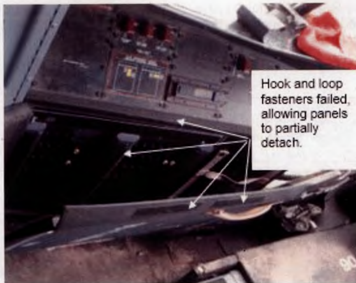
Figure 29 - Circuit Breaker Armour Panel partially detached.
