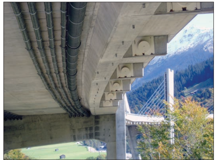
Fig. 15: Soffit of the bridge deck with ducts for wiring and sewage, de-watering drainage pipes and anchorages of the stay tendons (from left to right)
