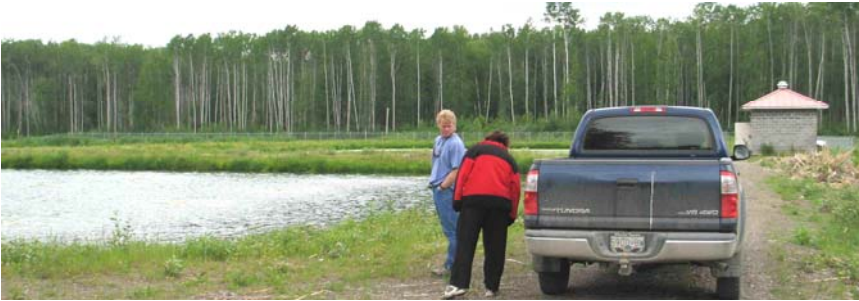
Figure 32. A secondary treatment lagoon at the Anderson Flats wastewater treatment plant.
