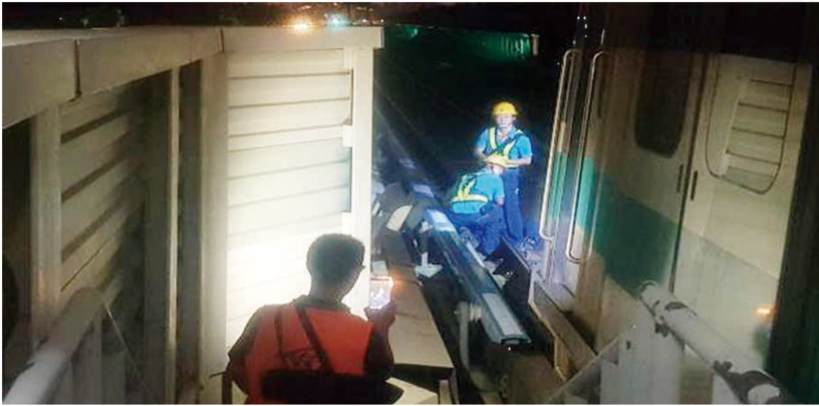
搶修人員拆除第三軌直流電纜 Repair personnel removing the 3rd rail DC cable
