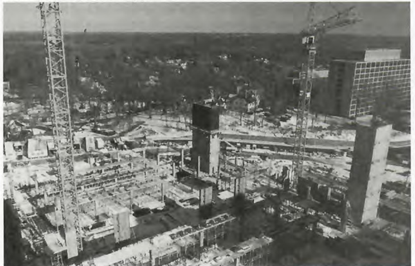
A thin blanket of snow covers the Mark O. Hatfield Clinical Research Center worksite just before Christmas. Officials say the site will soon swarm with more than twice as many workers as have appeared so far.
