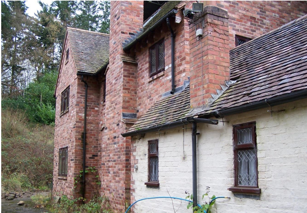
Rebuilt rear wing of Dowles – to be retained – rear of Barn Cottage in foreground
