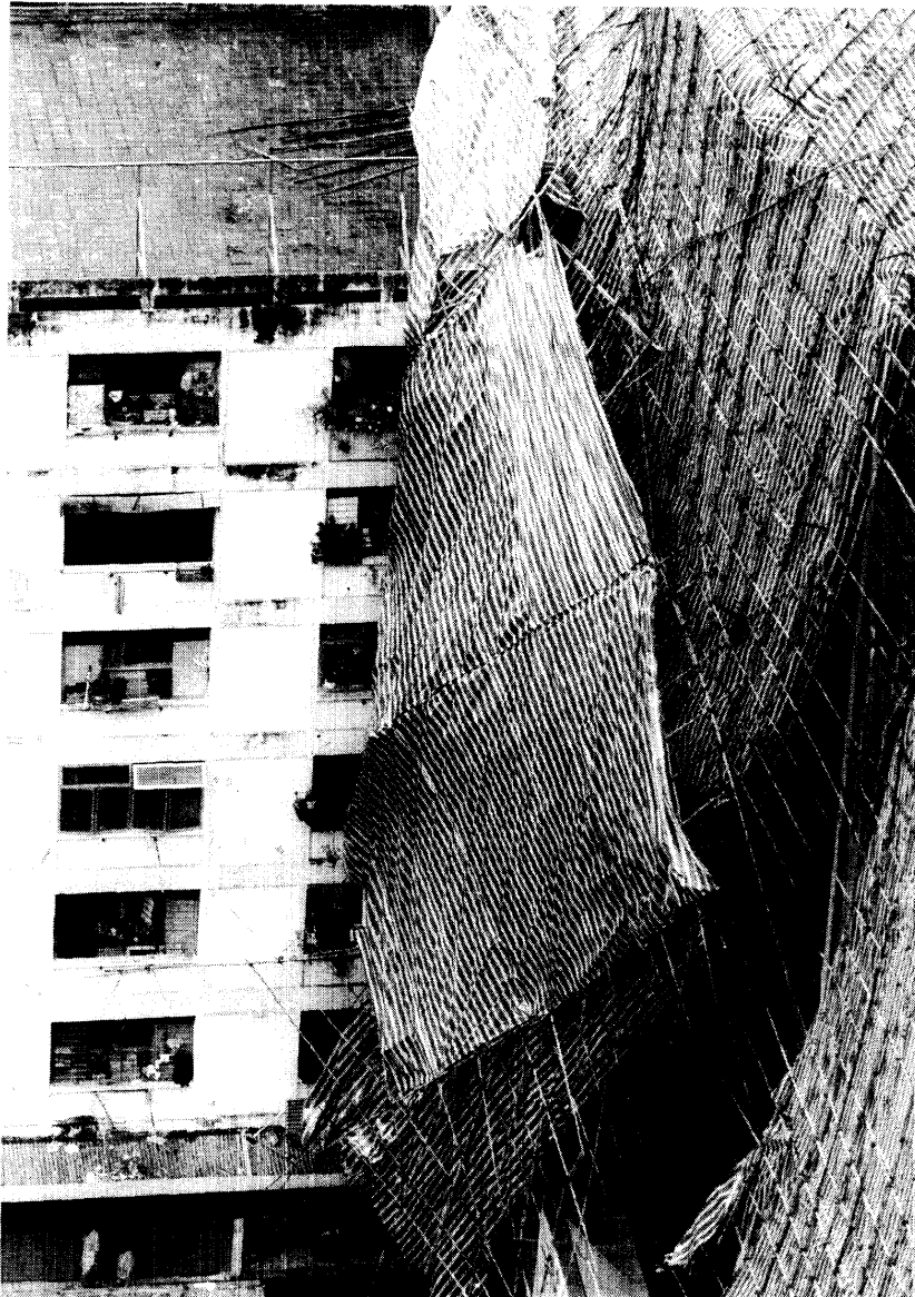
Figure 42. A large collapsed section of scaffolding in Shek Yam Estate, Kwai Chung (by courtesy of Sing Tao Daily).
